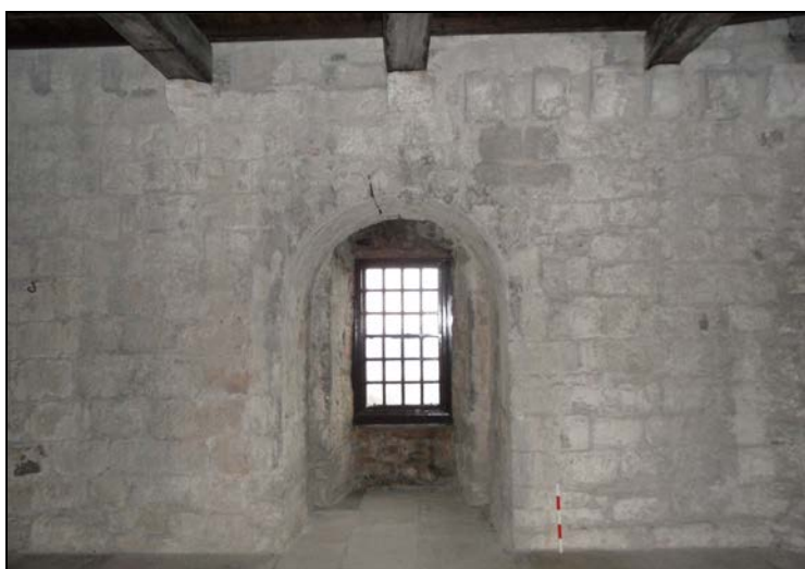
Plate 2.8: The break in build on the south wall on the 2 nd floor.
