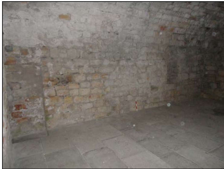
Plate 2.4: The break in build on the north wall and vault on the 1 st floor.
