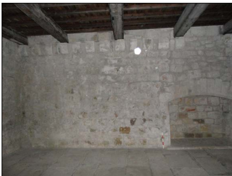
Plate 2.7: The break in build on the north wall on the 2 nd floor.
