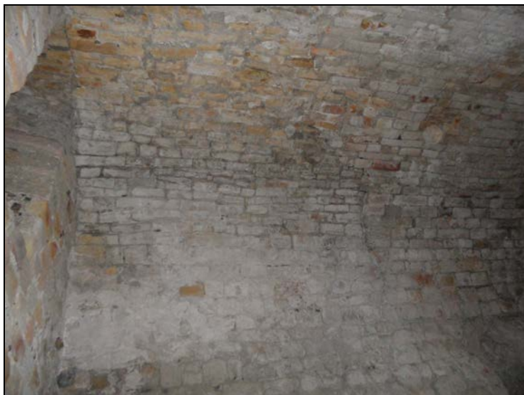
Plate 2.5: The break in build in the vault on the 1 st floor.
