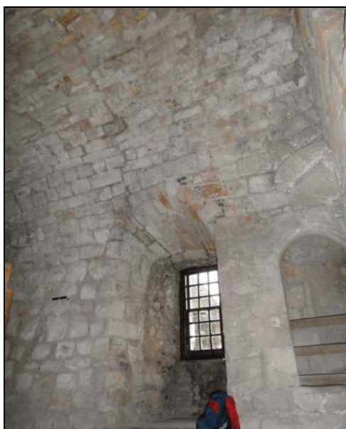
Plate 2.6: The break in build on the south wall and vault on the 1 st floor.
