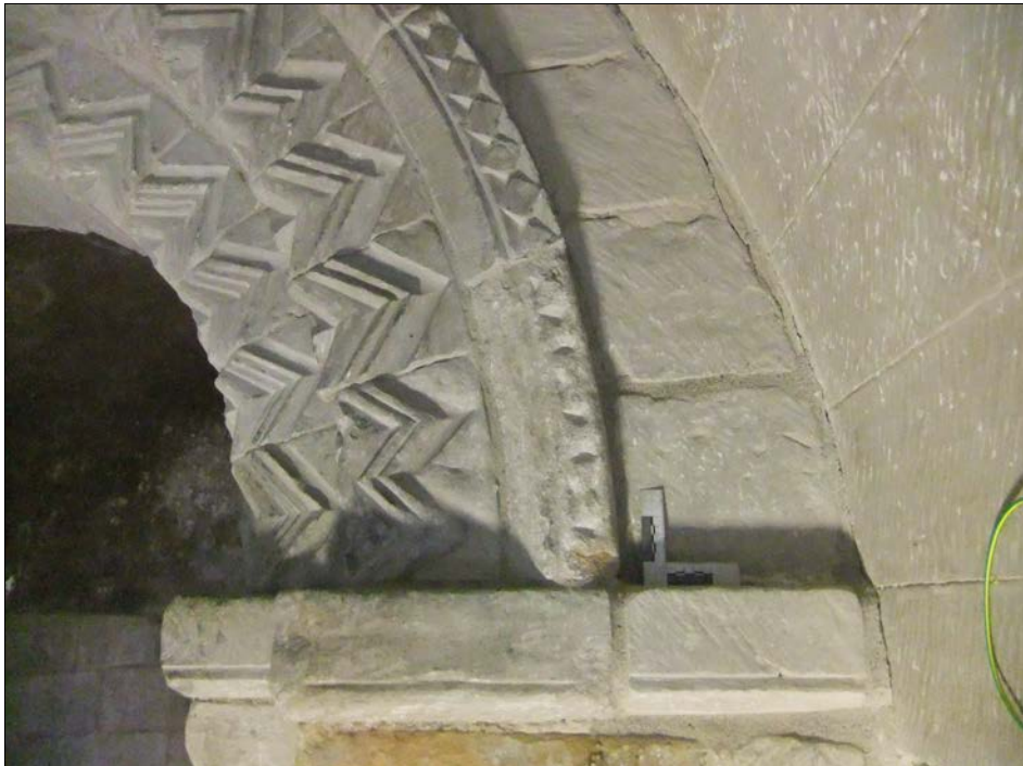
Plate 8: Detail of the base of the south end of arch 068, showing stone 065 and plinth 061.
