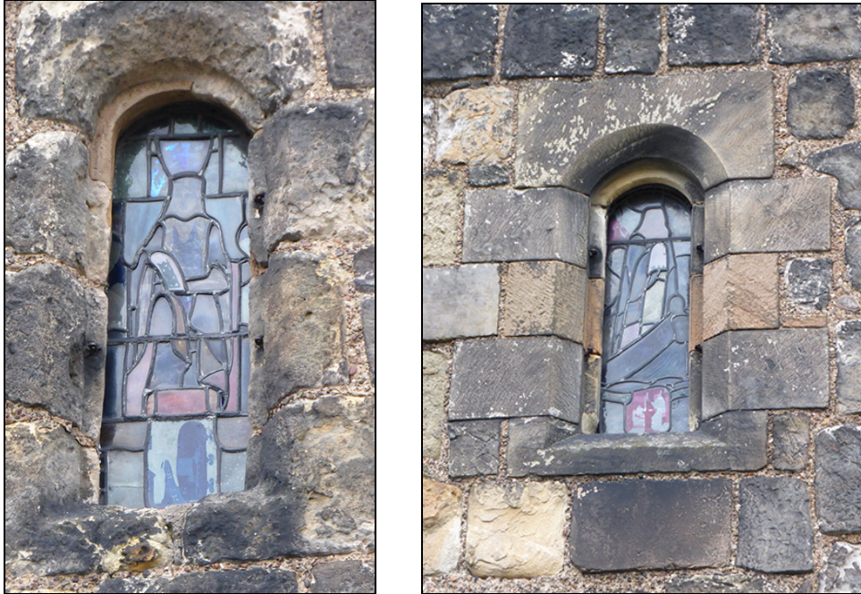
Plate 1: South windows of the nave. Left: unrestored west window, right restored east window.
