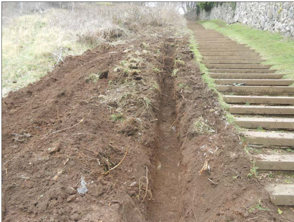
Plate 2: A view of the trench (with excavation in progress) adjacent to 'Jacob's Ladder'.
