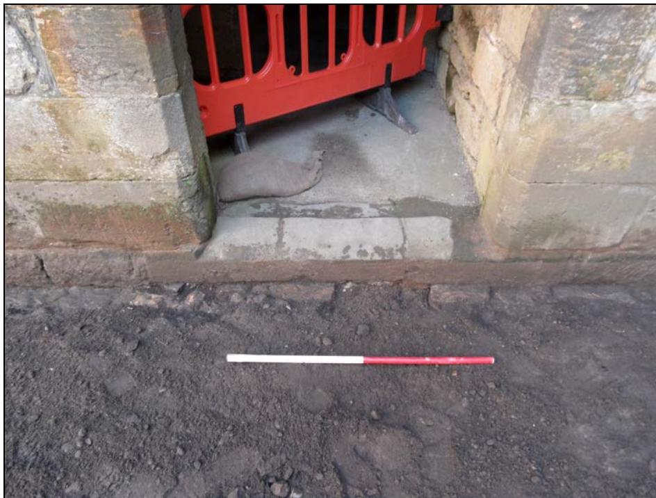
Plate 4: Looking east at the foundation course 302 of the east wall and the cut 309 through it.
