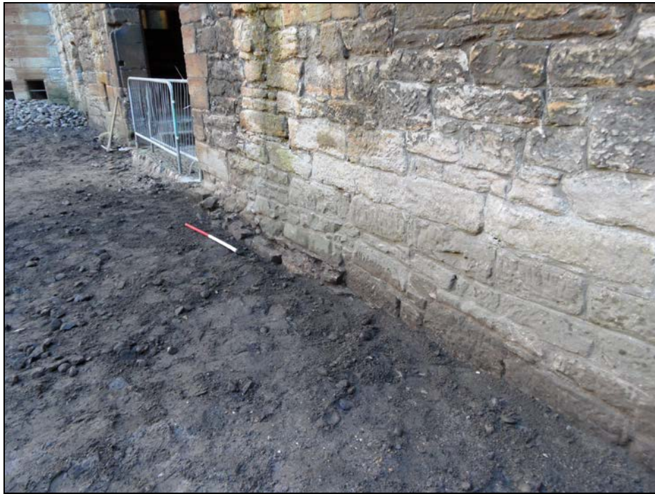
Plate 5: Looking north-east at the ragged foundation course 303 of the east wall at the east door.
