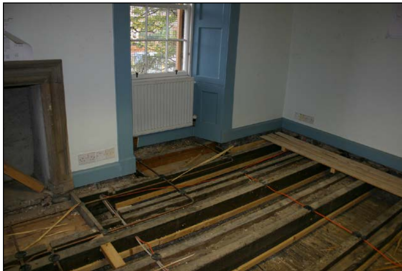
Nos. 009-011: View from northwest showing joist 009 and auxiliary joists 010-011 (second axis from left).
