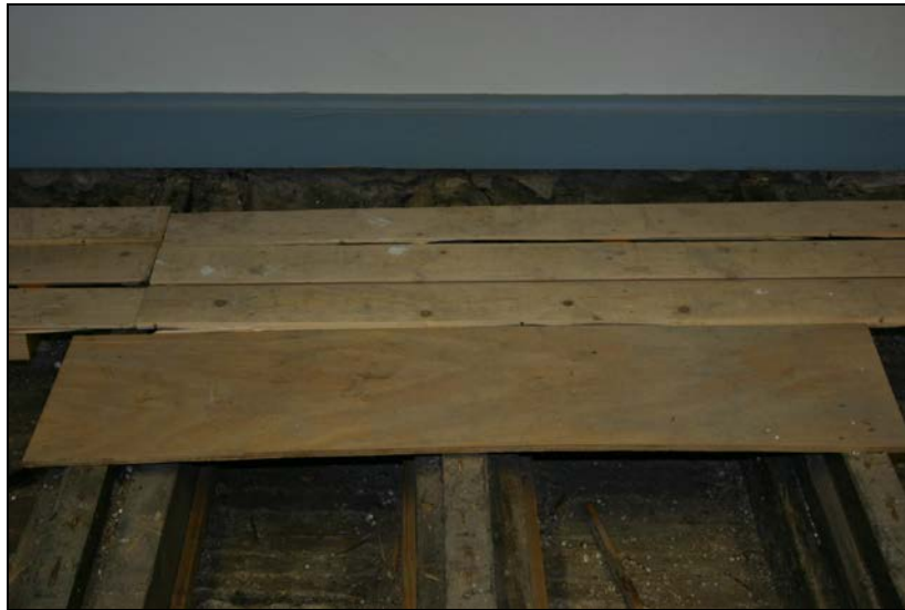
Nos. 023 and 024: View from north showing joist 023 and furring piece 024 (second axis from left).
