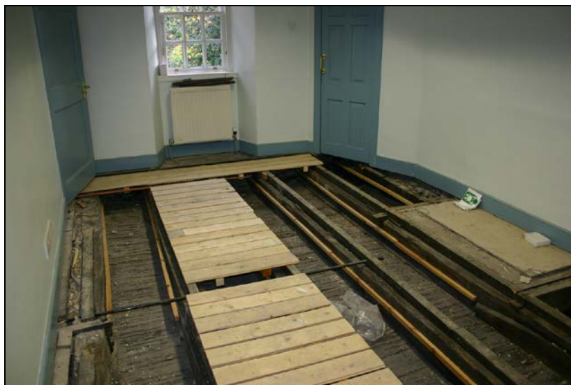
Nos. 066 and 067: View from north showing joist 066 and furring 067 (fourth axis from left).
