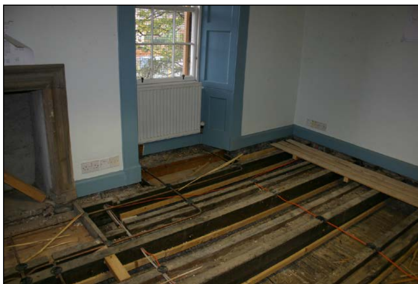
Nos 003, 004 & 008: View from north-west showing joist 003, auxiliary joist 004 and trimmer 008 (first axis in front of e-wall).
