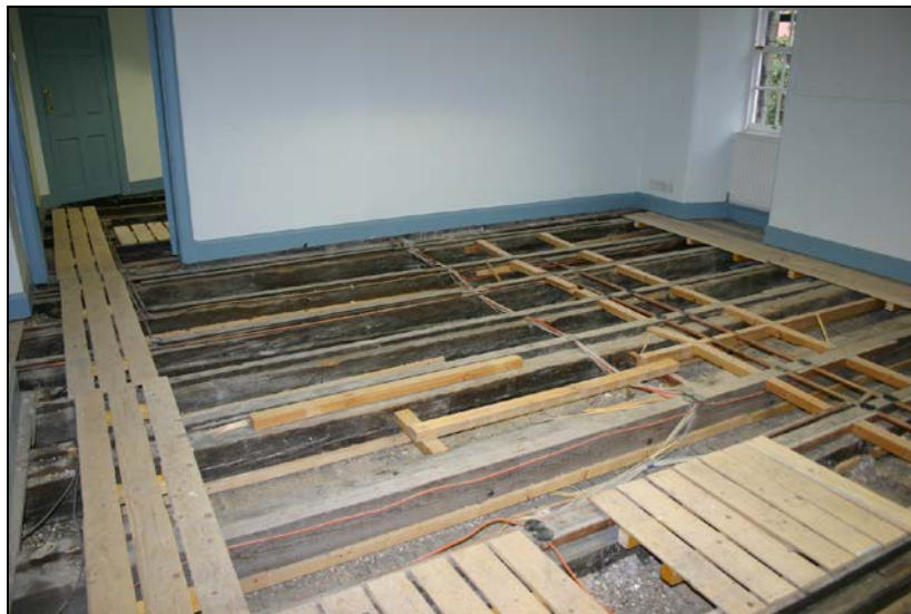
Nos. 041 and 042: View from southeast showing joist 041 and furring 042 (fourth axis from left).
