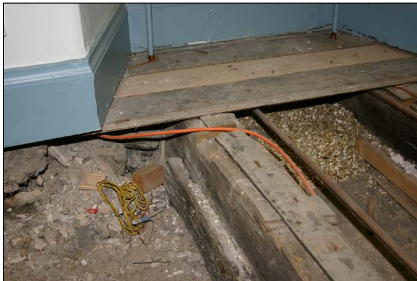
Nos. 047, 048 and 049: View from south showing joist 047, furring 048 and auxiliary board 049 (second axis from right).
