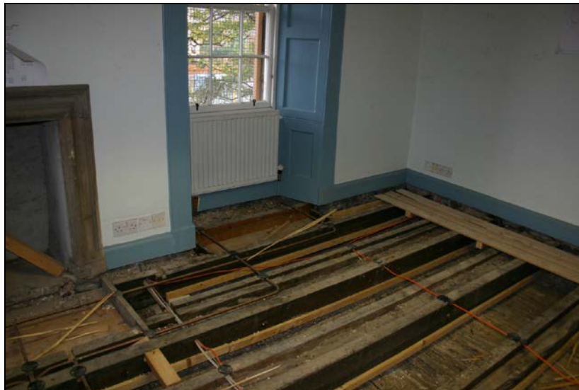
Nos. 015-017: View from northwest showing joist 015 and auxiliary joists 016-017 (third axis from left).
