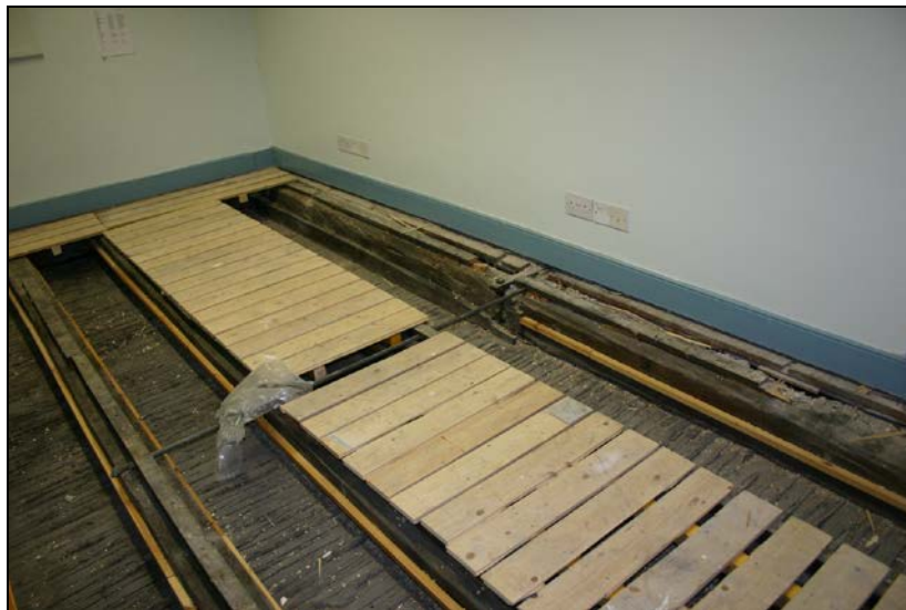
Nos. 060 and 061: View from southwest showing joist 060 and furring 061 (second axis from right).
