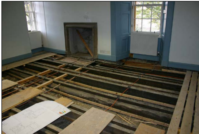
Nos. 018 and 019: View from northeast showing joist 018 and furring piece 019 (third axis from right).
