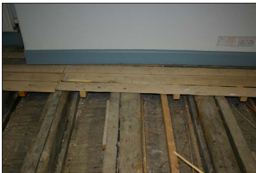
Nos. 038 and 039: View from south showing joist 038 and auxiliary joist 039 (second axis from left).
