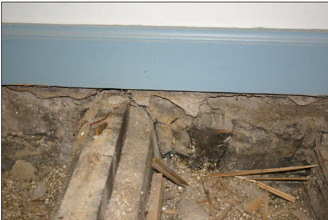
Figure 5: Redundant joist-stumps adjacent to joist 023.
