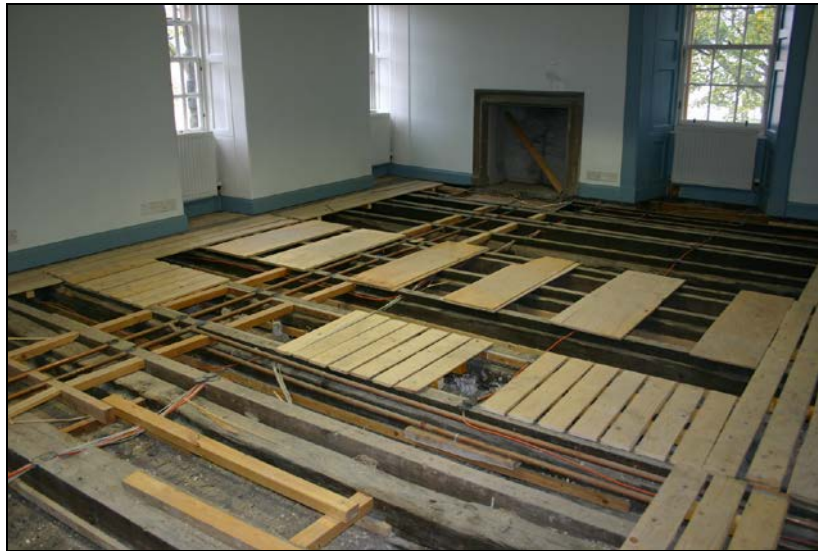
Nos. 028 and 029: View from northwest showing joist 028 and furring 029 (second axis from left).
