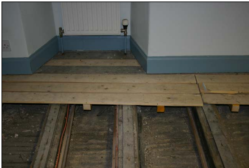
Nos. 044, 045 and 046: View from south showing joist 044, furring 045 and auxiliary board 046 (second axis from left).
