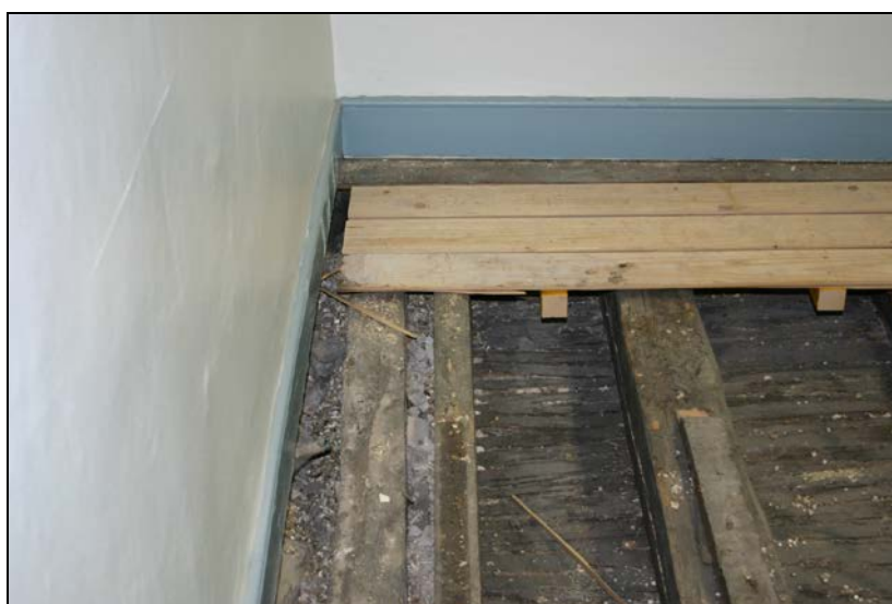
Nos. 073 and 075: View from south showing joist 073 and auxiliary joist 075 (first axis from left).
