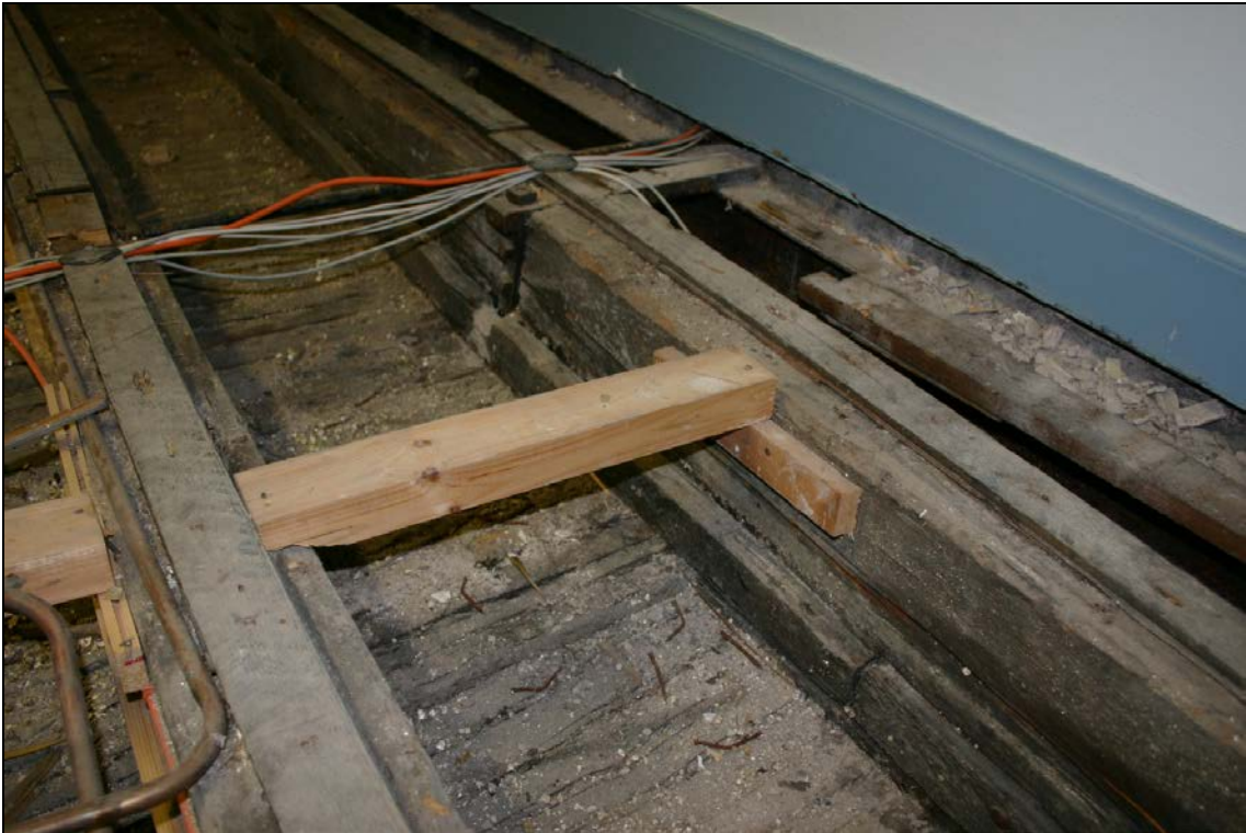
Figure 9: Iron bracket and partition at joist 050.
