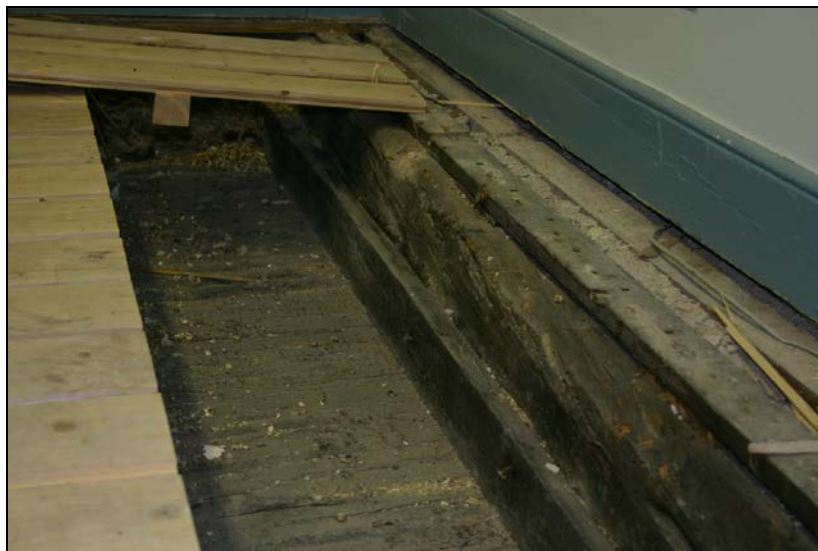
Nos. 057, 058 and 059: View from southwest showing of joist 057, furring 058 and auxiliary board 059.
