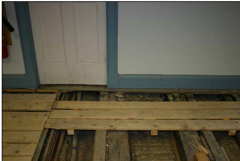
Nos. 033 and 034: View from north showing joist 033 and auxiliary joist 034 (second axis from right).
