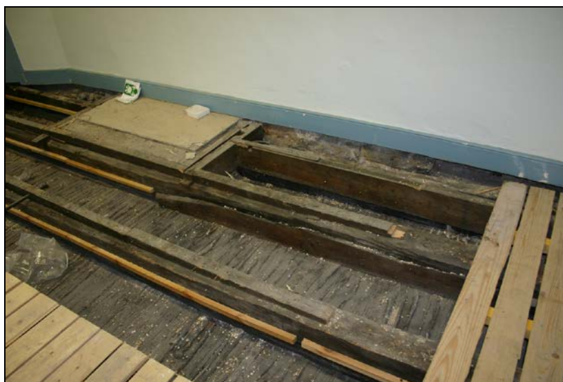
Nos. 069, 070, 071, 075 and 076: View from northeast showing joist 069, furring 070, auxiliary board 071 and trimmers 075 and 076 (second axis from right).
