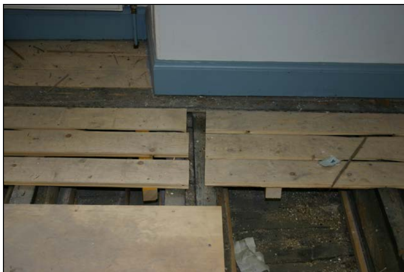
Nos. 020-022: View from south showing joist 020, auxiliary joist 021 and furring piece 022 (second axis from left).
