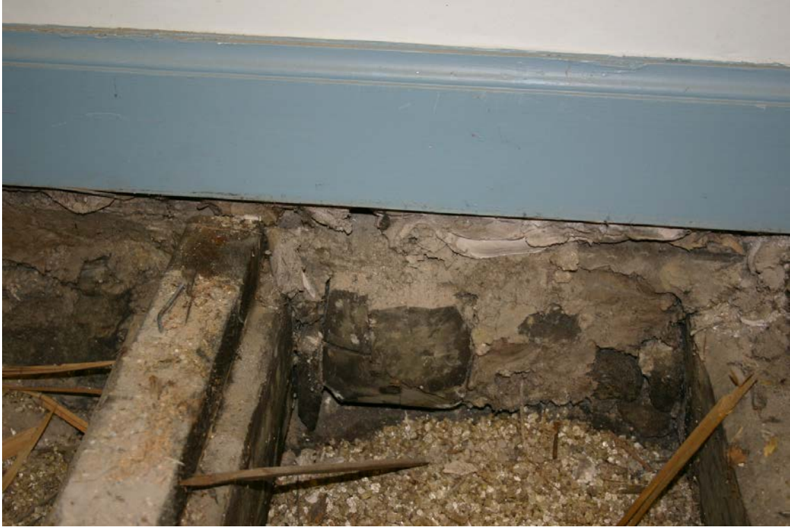
Figure 6: Redundant joist-stumps adjacent to joist 025.
