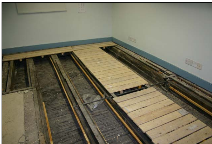
Nos. 063 and 064: View from southwest showing joist 063 and furring 064 (third axis from right).
