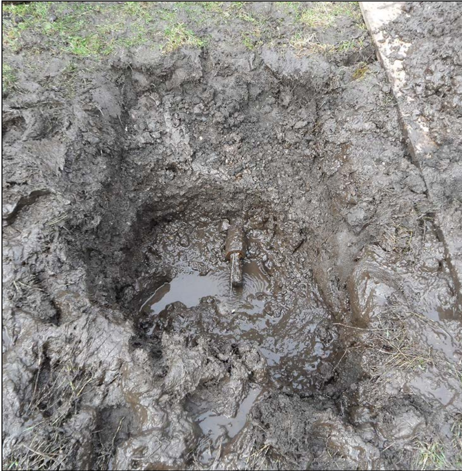
Plate 1: A view of pipe 103 with leaking plug 104 exposed, from the south-east.
