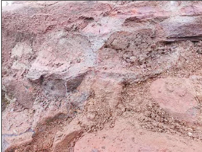
Plate 2: The hard grey cement atop the historic wall fabric
