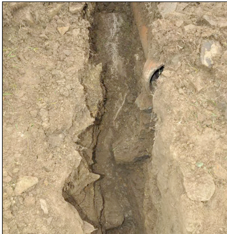
Plate 1: The masonry 004 at the bottom of the trench. The pipe (005) is visible to the right.
