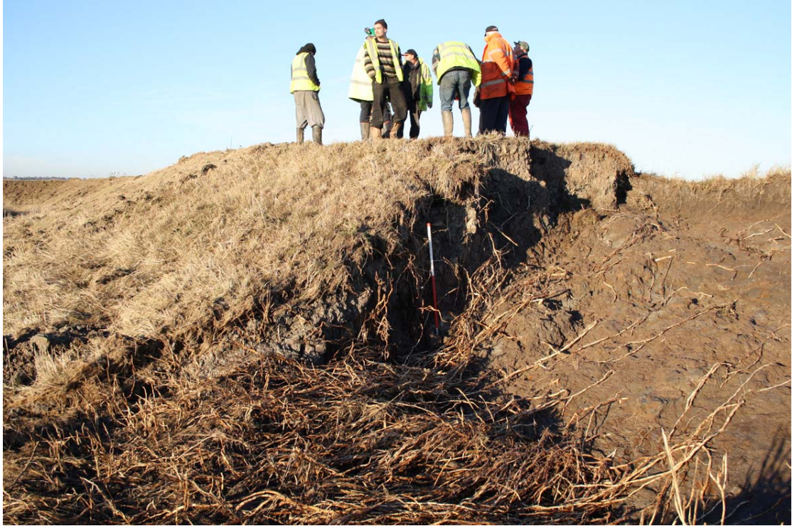
Plate 1. Showing breach in sea wall, looking north-west.
