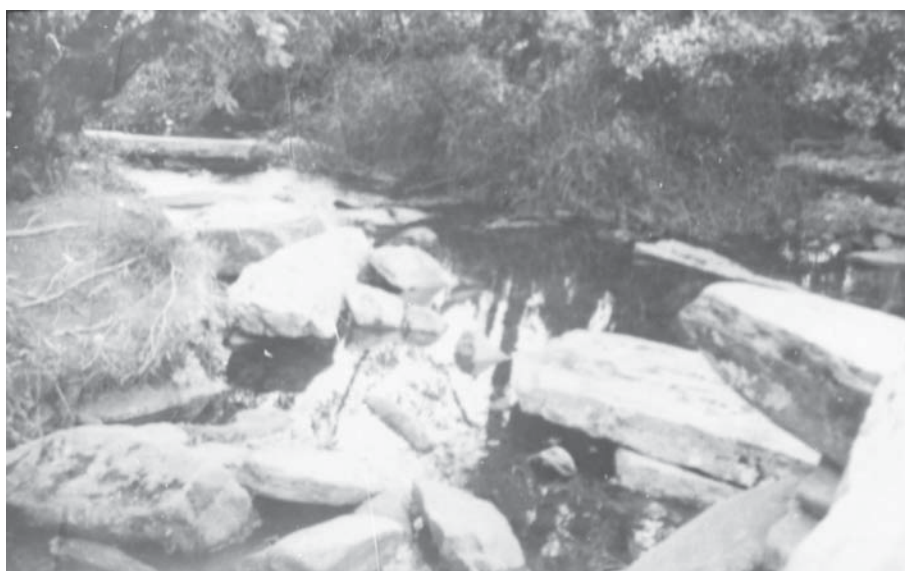
Fig 23 Damage to Tarr Steps, late 1939 (SRO county neg no 10515)
