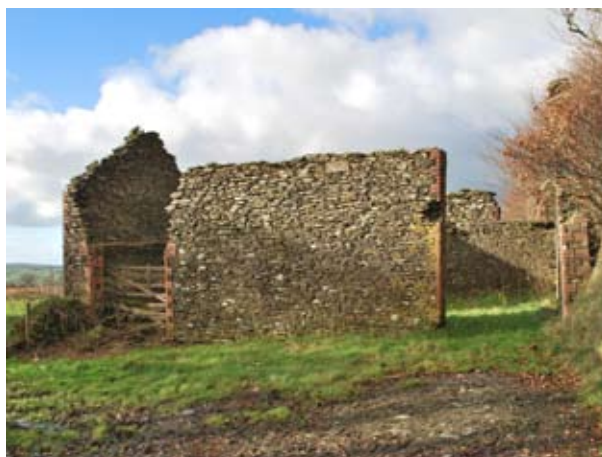
Fig 20 (right) The SE side of the linhay (BFD17008) on Fullaford Down (1m scale) (Hazel Riley)
