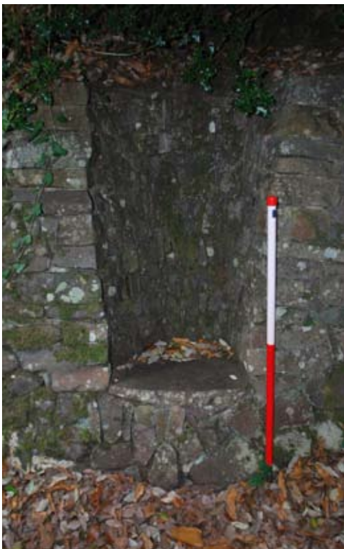
Fig 52 (below) Recent rebuilding of the 19 th -century arboretum wall (1m scale) (Hazel Riley)
