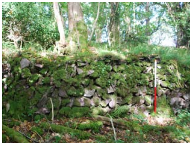
Fig 53 (left) Recent modifications to the retaining wall to create a seat, Drive 1 (1m scale) (Hazel Riley)
