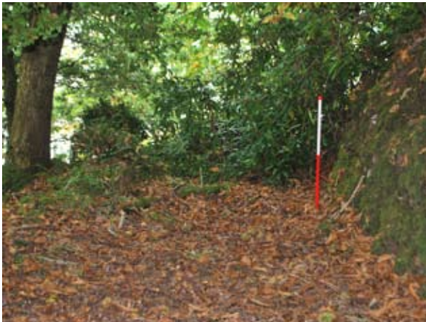
Fig 38 (left) Drive 3 destroyed by landslip, west of Ashley Combe (1m scale) (Hazel Riley)
