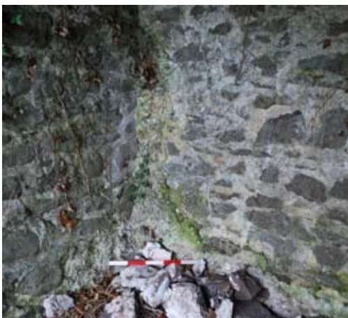
Fig 18 (below) Lime in the southern corner of the lime store (0.5m scale) (Hazel Riley)
