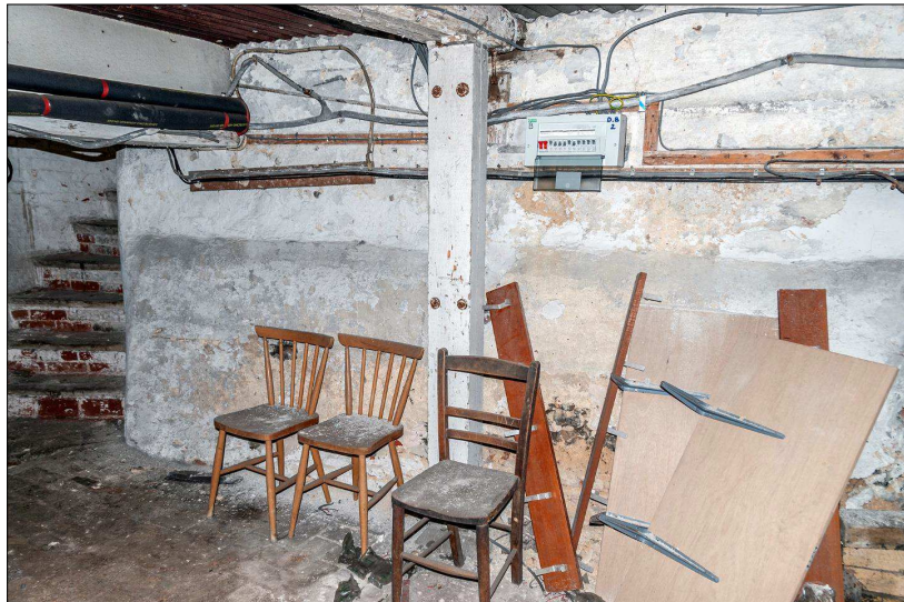
Plate 3. North wall of cellar below No.71, incorporating remains of the north wall of the medieval bell tower. (Photo by Dr R.B.Harris, 2007)
