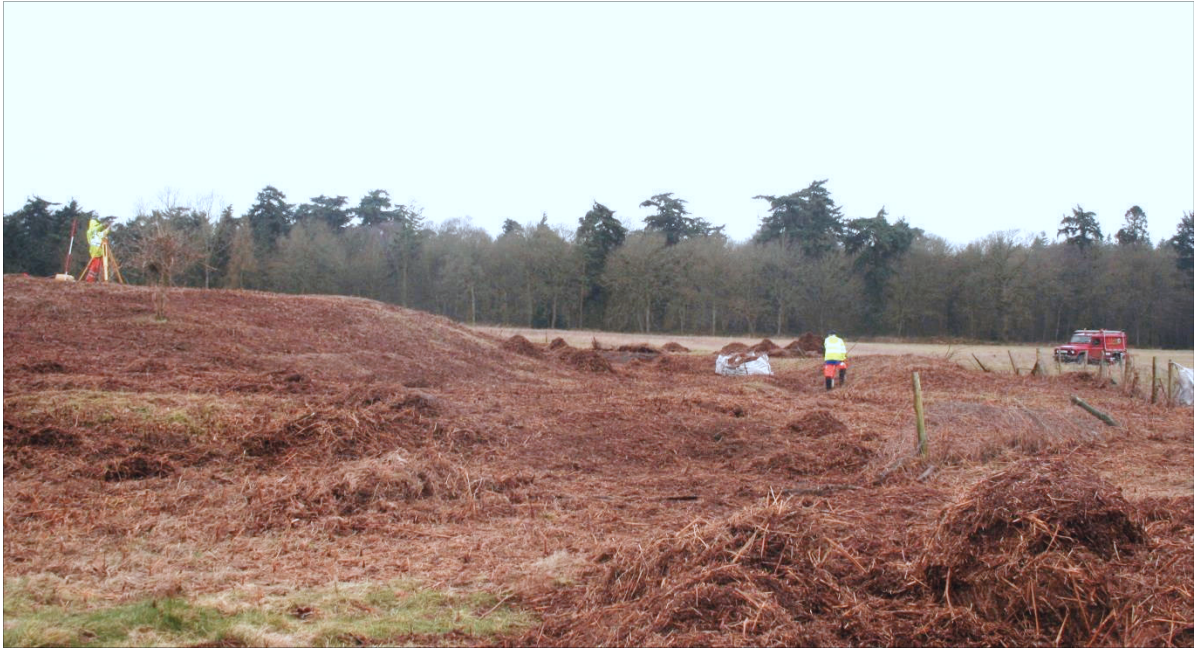
Plate 5: Clearance of the north part of the Barrow in progress. (looking W)
