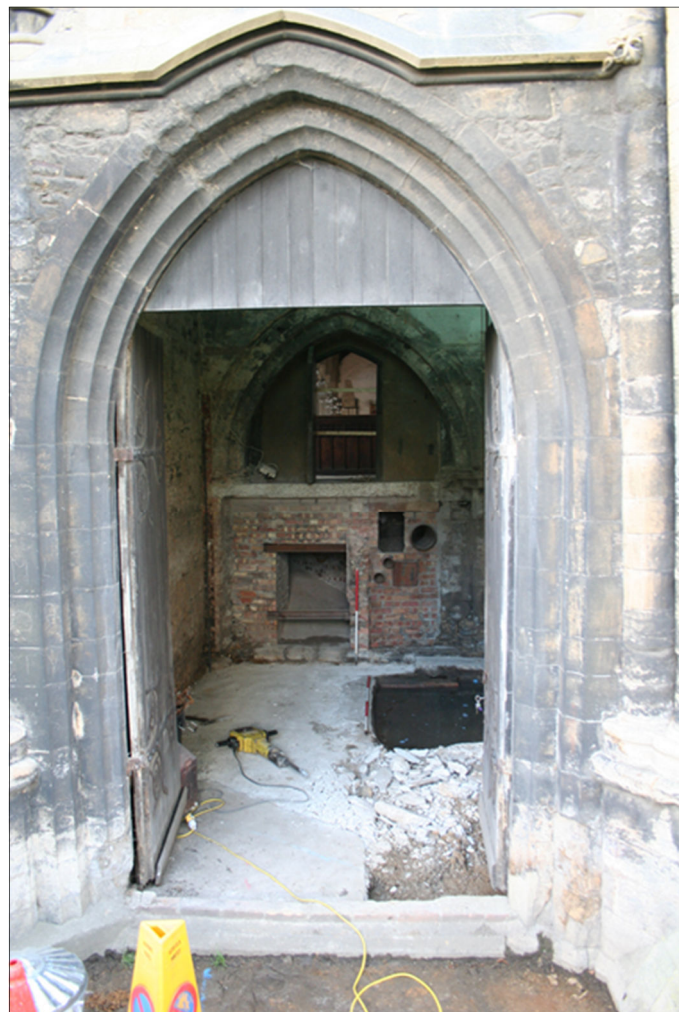
Plate 20: View into the tower (concrete floor in place) looking E) [1x1m & 1x2m Scales]
