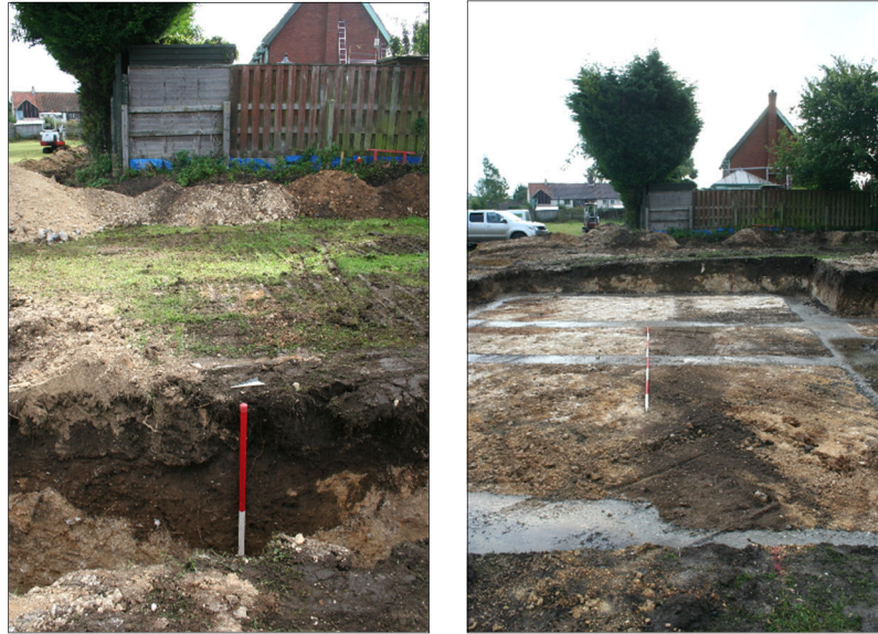
Plate 7 & 8. Plot 3: Ditch [12] profile [1x1m Scale] + in plan post-overburden reduction [1x4m Scale] (both looking E)
