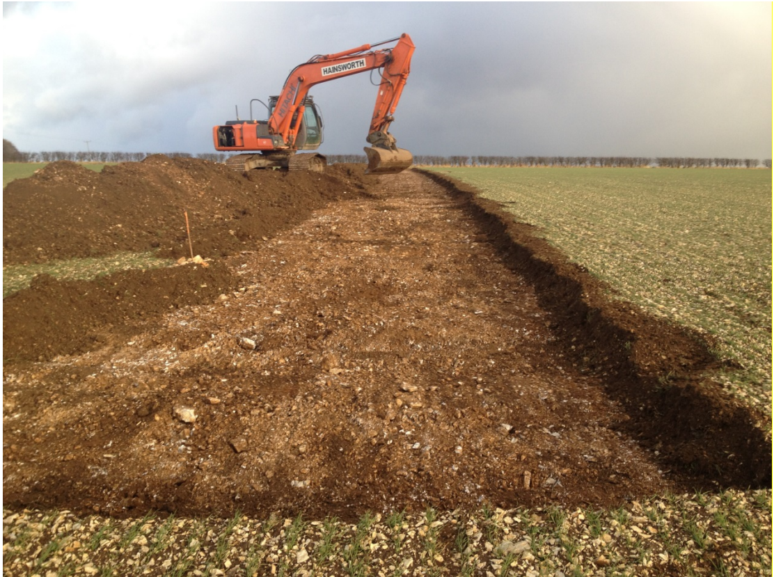
Fig. 3 Stripped access track looking north-east from the turbine location back towards the field boundary.
