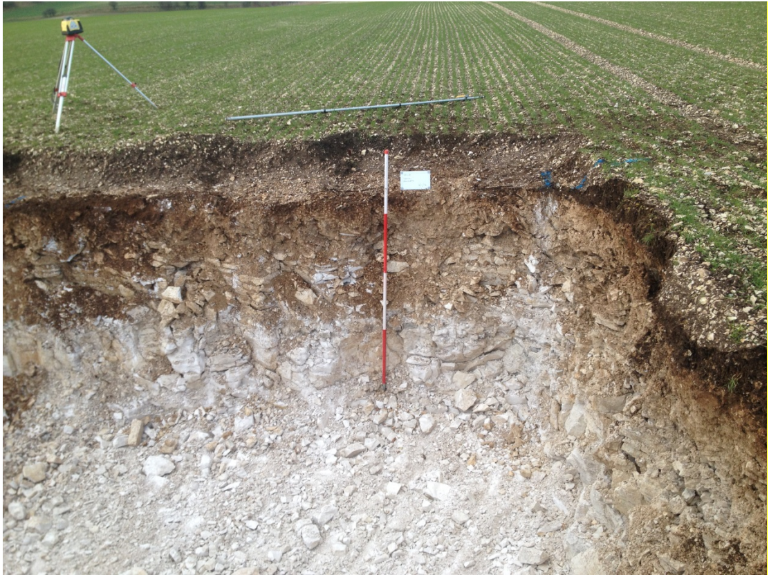
Fig. 4 Fully excavated pit for turbine base showing the thin overburden overlying chalk brash and bedrock.
