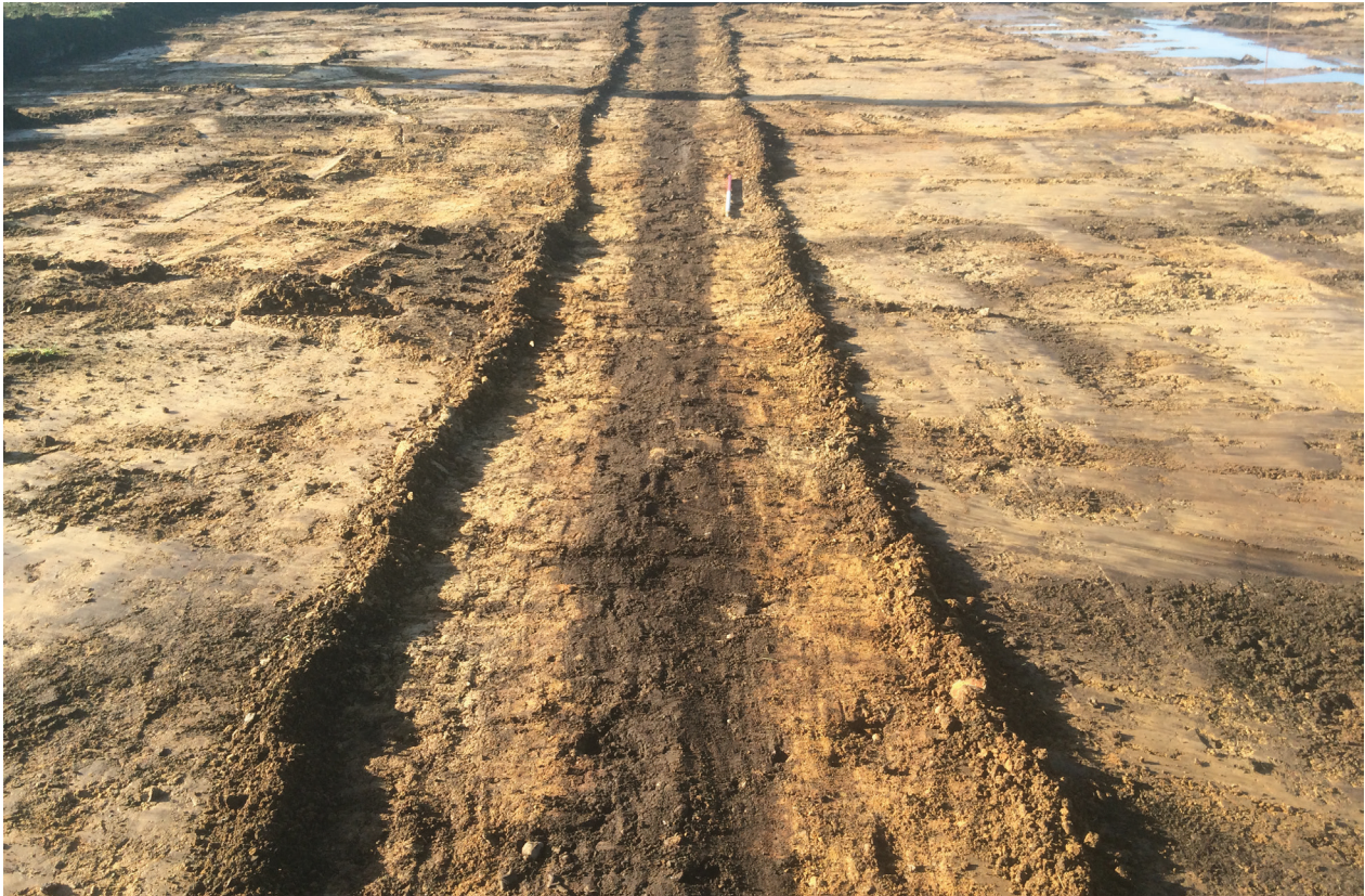
Fig. 5 Modern field drain F014 looking south-west across the open area of the turbine base and crane pad (scale 1m)
