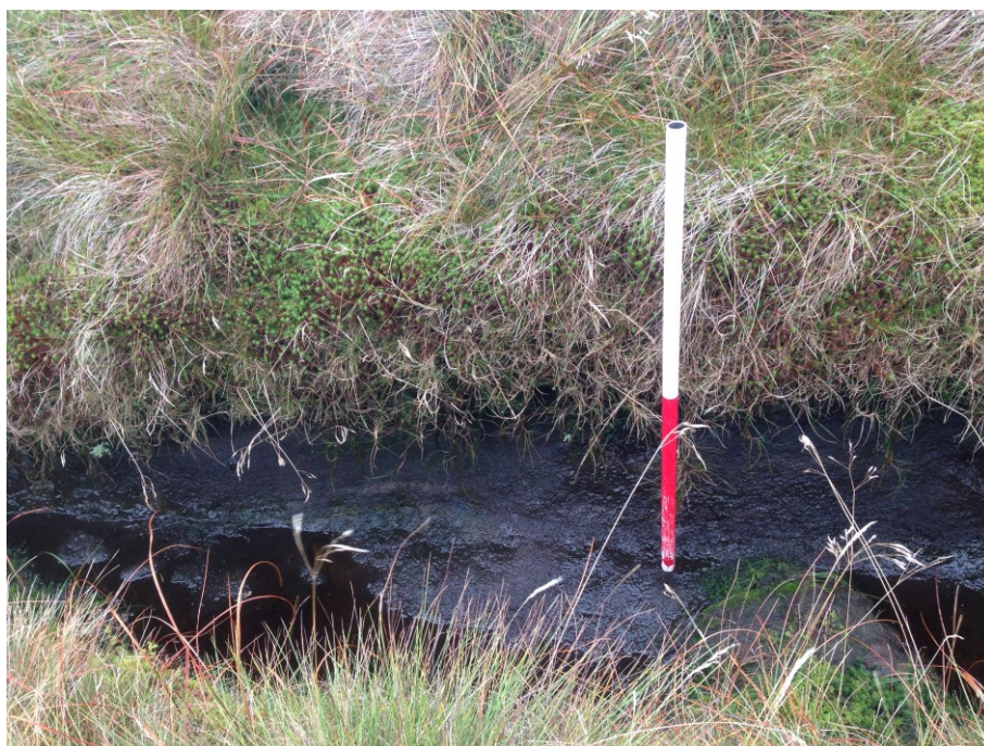
Figure 4 Example of one of the 20 th -century grips within the survey area showing the depth of peat exposure (scale = 1m).
