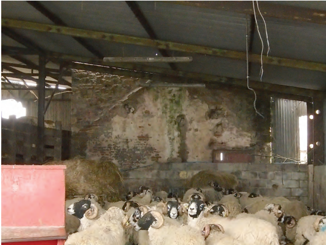
Figure 72 Building B, west elevation of two-storey barn. Note raggle of previous roofline for single-storey extension. No scale
