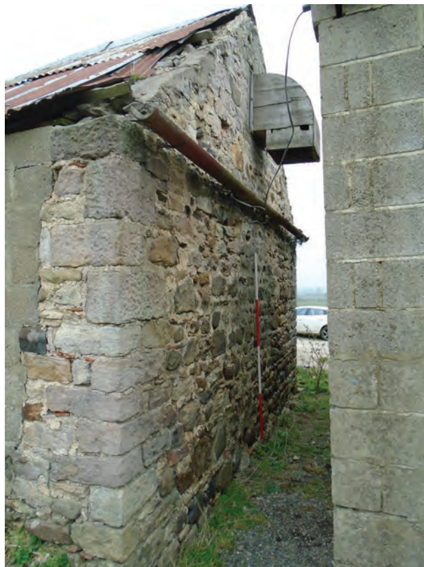
Figure 67 Building B south elevation of southern extension, facing east. Scale 1x2 m
