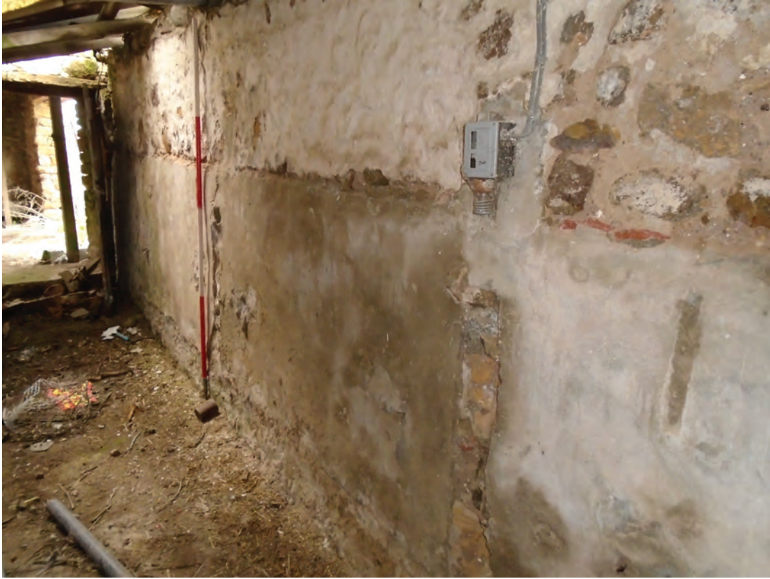
Figure 76 Building B, Room G1, detail of east wall, looking north-east. Scale 1x2 m
