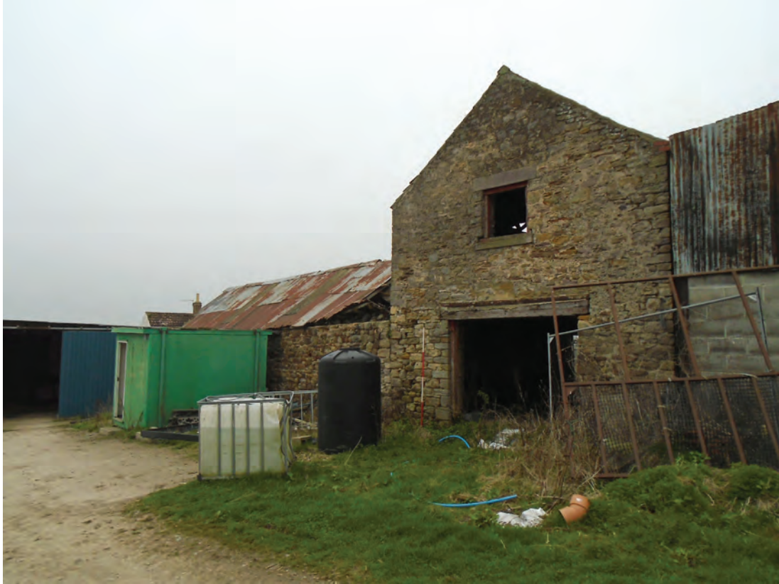
Figure 70 Building B, north extent of east elevation. Note clear construction break between two phases of development. Scale 1x2 m
