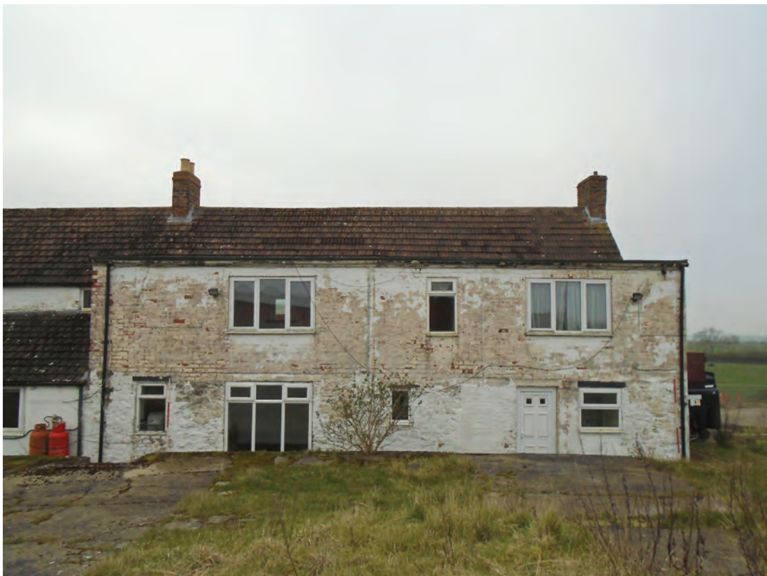
Figure 9 West extent of north elevation of Building A, facing south. Scale 2x2 m
