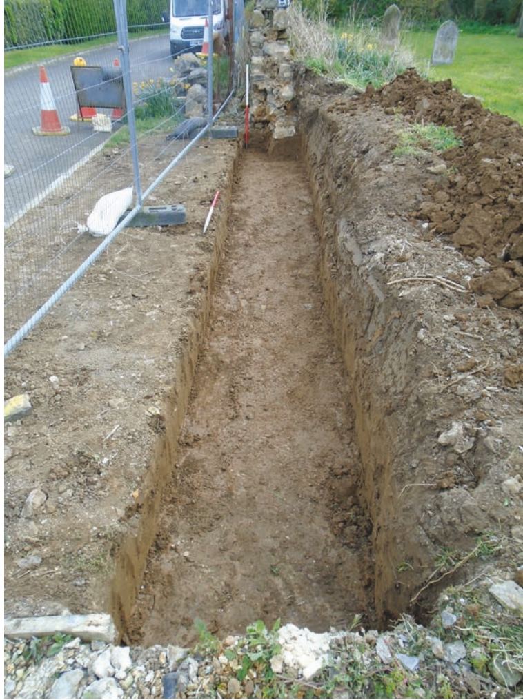
Figure 7 New foundation trench for northern section of rebuilt wall, looking east. Note old wall sitting on clay till substrate. Scale 2x1 m
