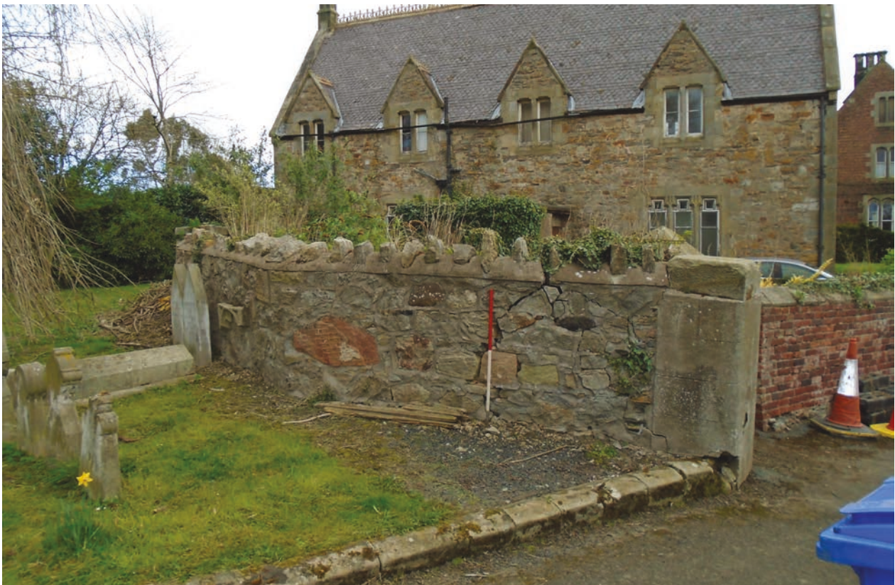
Figure 3 Failing section of wall adjacent to the entrance to the churchyard from Main Street, prior to the commencement of works, looking north-east. Scale 1x1 m
