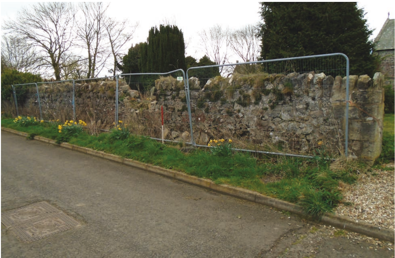
Figure 6 Failing length of wall at the north side of the churchyard, adjacent to Church Lane, prior to the commencement of works, looking south-east. Scale 1x1 m
