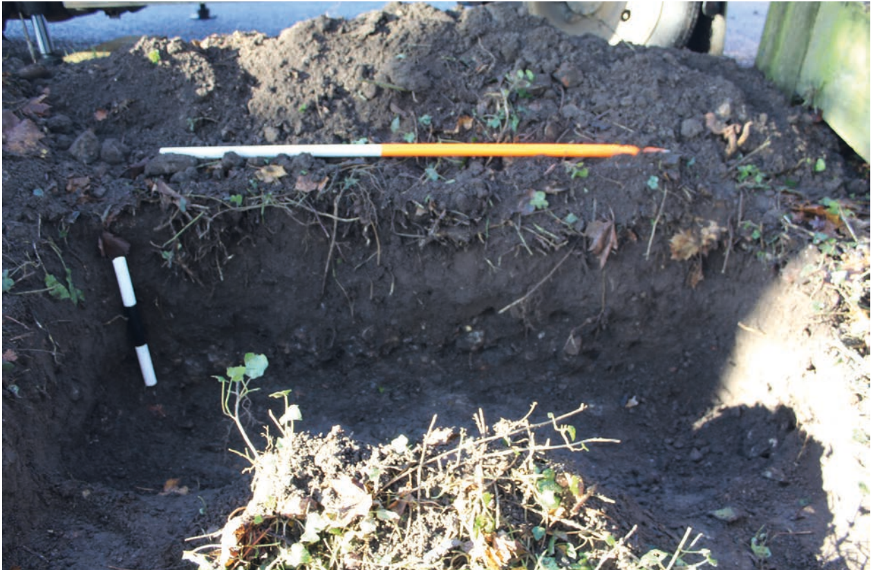
Figure 3 Western bridge footing excavation facing west. The bedding deposit for the adjacent road can be seen at the base of the facing section. Scales = 1 m and 0.3 m
