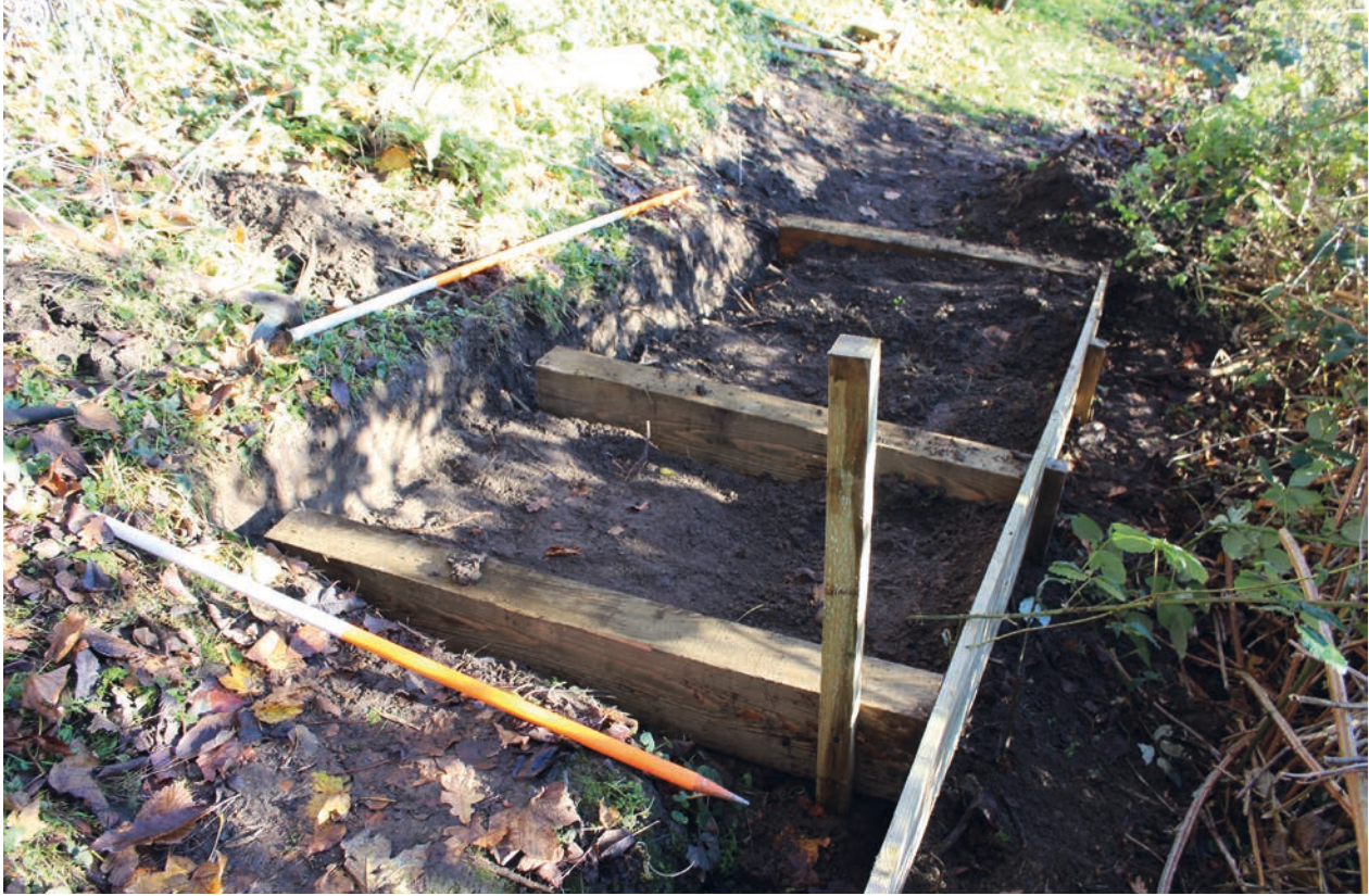
Figure 5 Overall view of the footpath trench following excavation and insertion of the wooden boards. The angle of excavation shows the cut into the bank to the left of shot and the filled material to the right-hand side of the excavation. Scales = 1 m and 2 m
