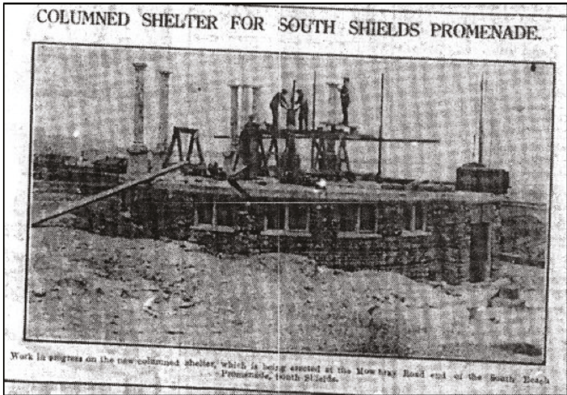
Figure 2 Photograph of work in progress on the new columned shelter being erected at the Mowbray Road end of the South Beach Promenade. From The Shields Daily Gazette and Shipping Telegraph (The Shields Gazette), published 1st July 1931
