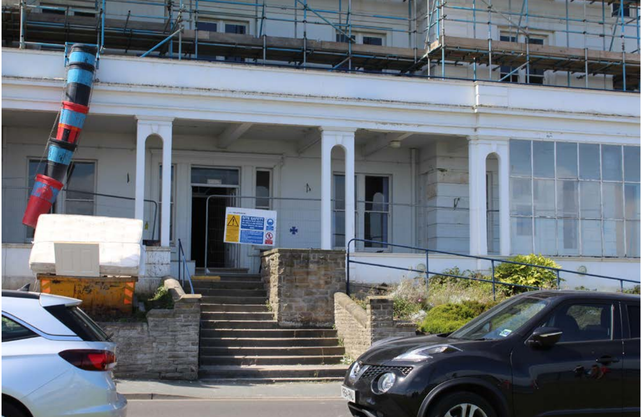
Figure 4 Narrowed stone stairs and disabled access ramp railing
