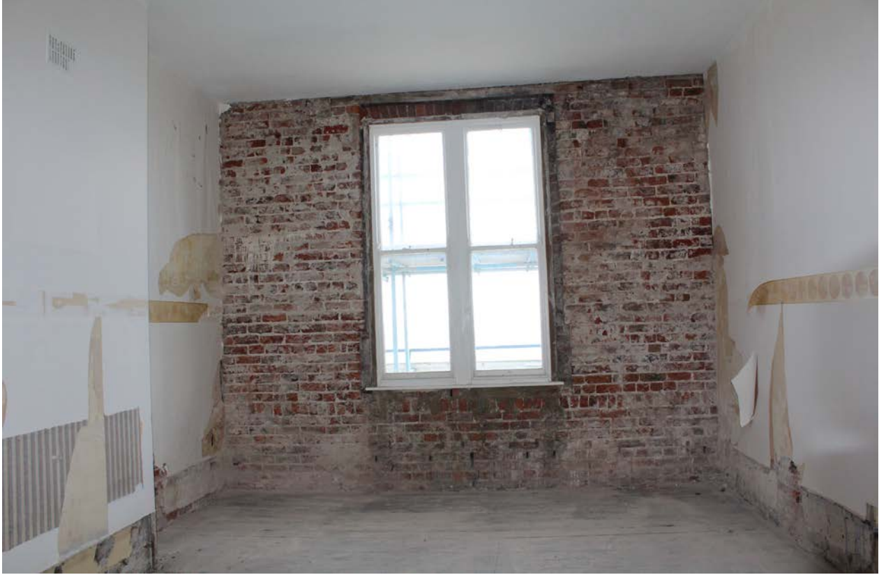
Figure 15 Example of unsympathetic modern replacement glazing
