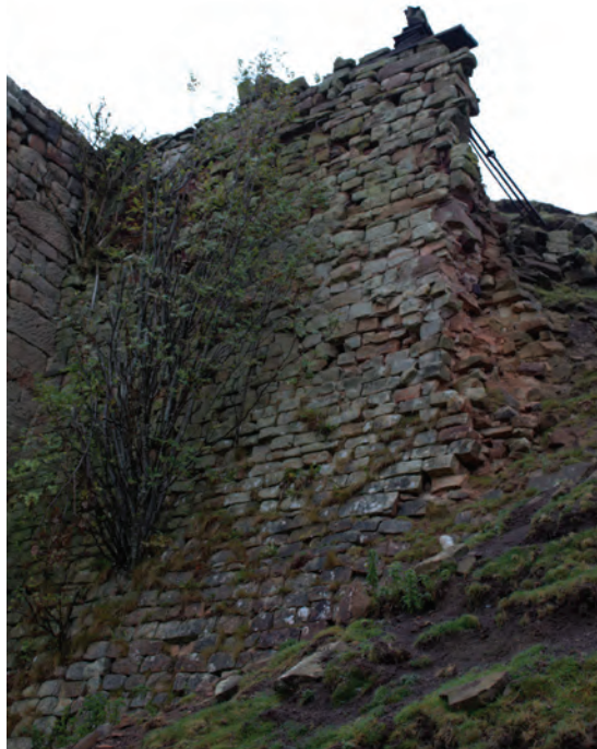
Figure 6 Area of work at south side of Pier 3 prior to commencement of work, looking north east. No scale
