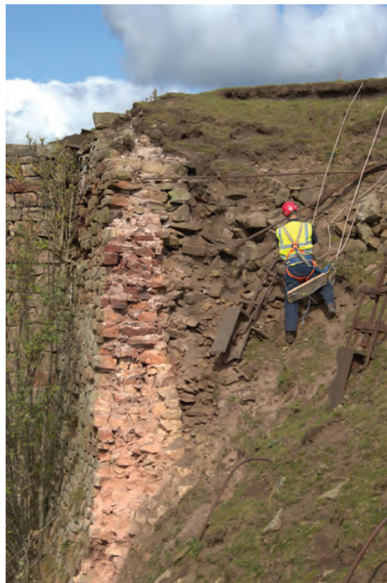
Figure 8 Work area at south side of Pier 3 at completion of the works, looking north
