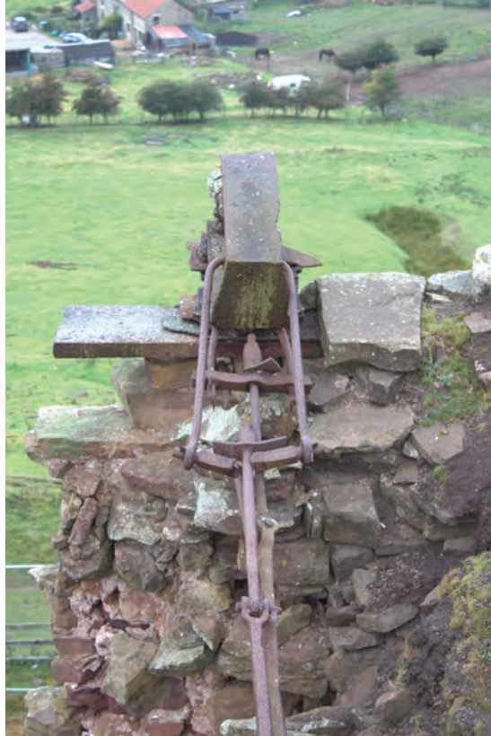
Figure 4 Arrangement of adjusting bolts and articulating joints to rear of tie beam at south side of Pier 3, looking west. No scale
