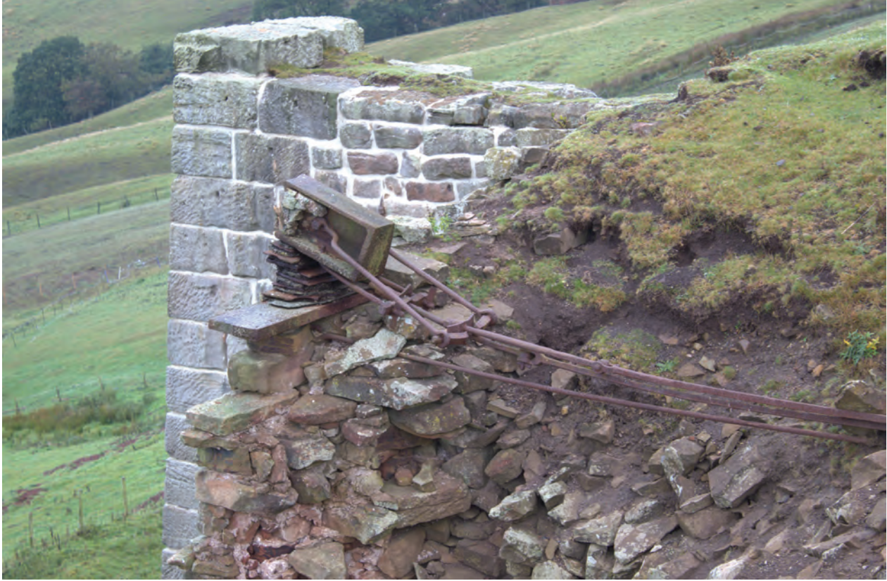
Figure 3 Location and arrangement of tie beam structure at south side of pier, prior to commencement of work, looking north-west. No scale
