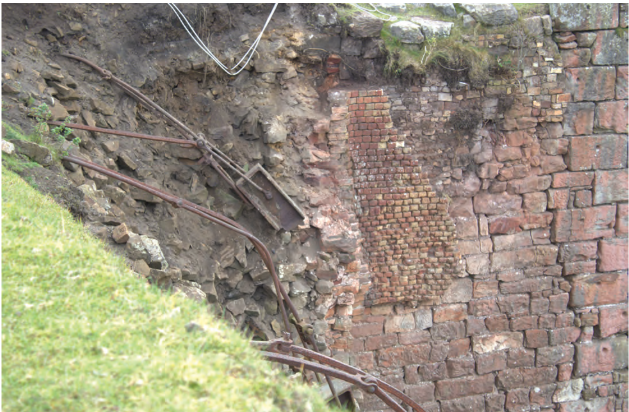
Figure 12 Area of work at north side of Pier 3 following completion of the works. No scale
