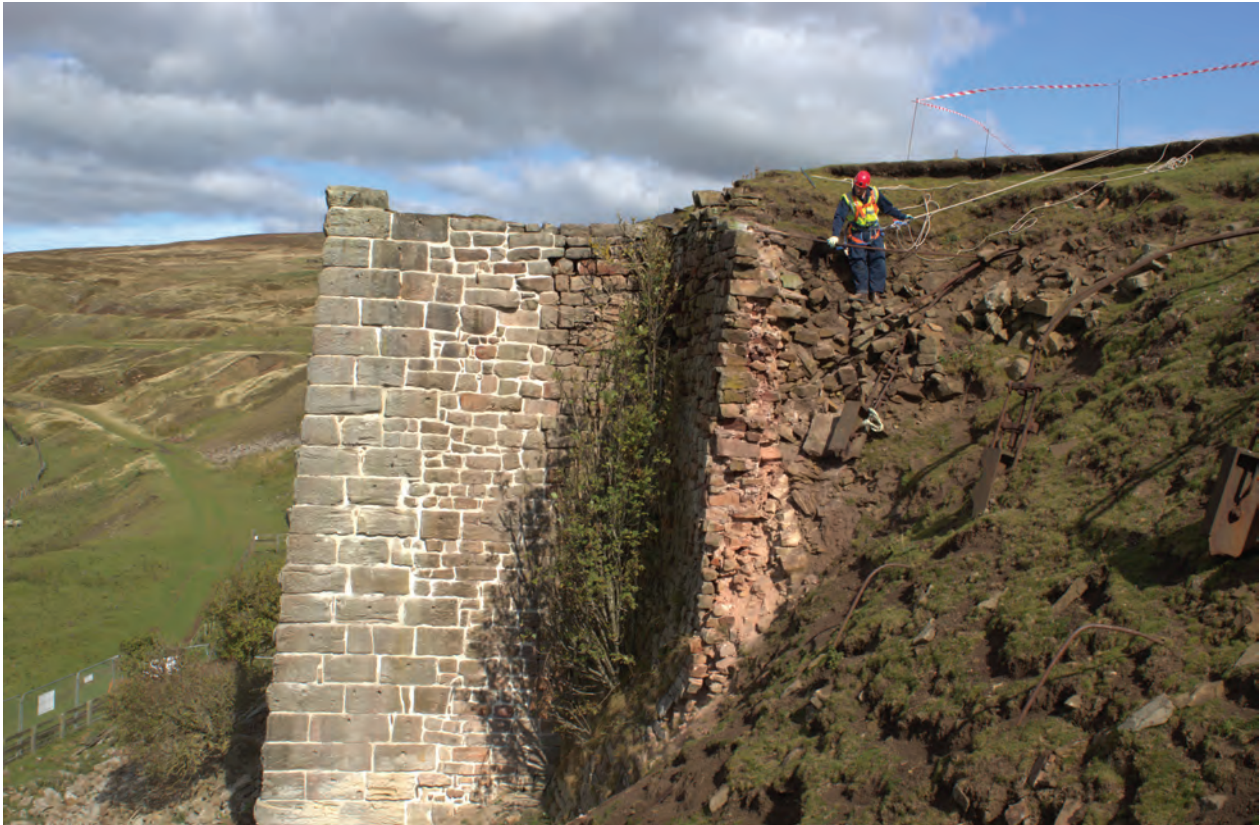
Figure 7 Takedown works being carried out to the south side of Pier 3, looking north
