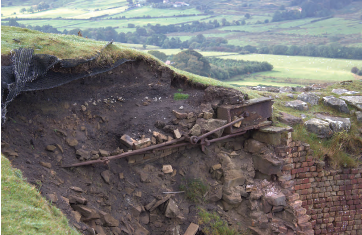
Figure 10 Detail shot of tie beam surrounded by firebrick brickwork behind the rear kiln wall, looking south-west. No scale
