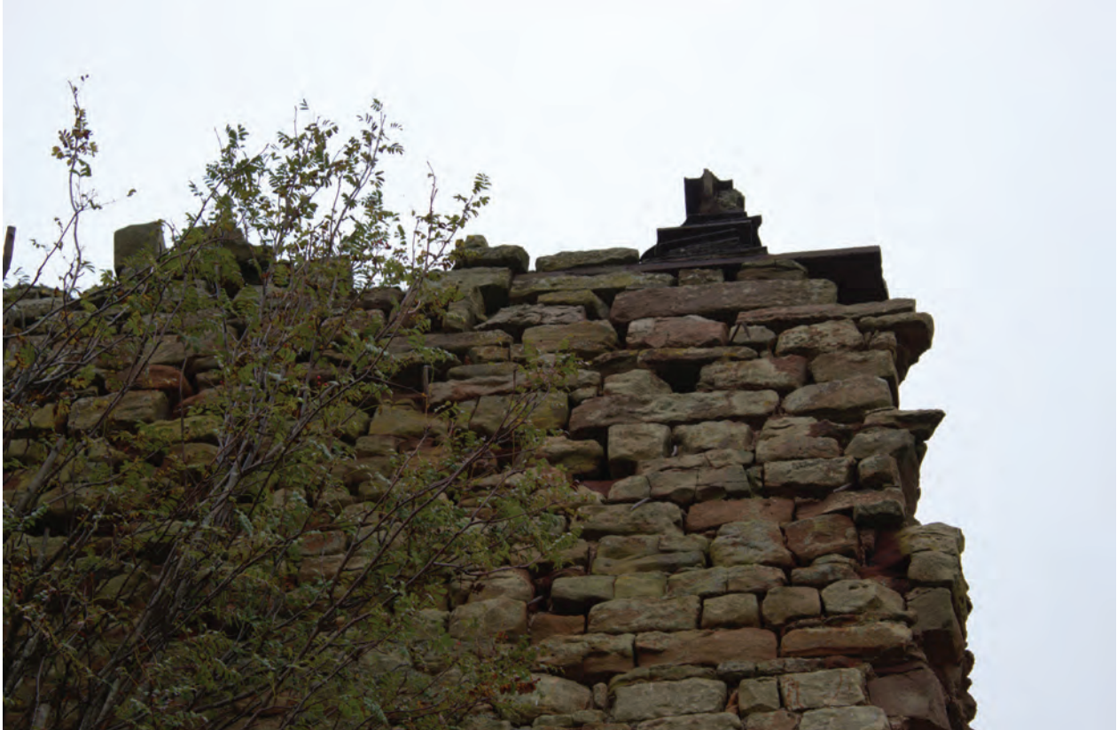
Figure 5 Detail of upper section of rear kiln wall prior to work commencing. Note thin wrought iron ties protruding from wall face at upper right. No scale
