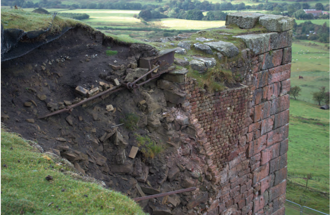
Figure 9 Area of work to north of Pier 3, prior to commencement of works, looking south-west. No scale
