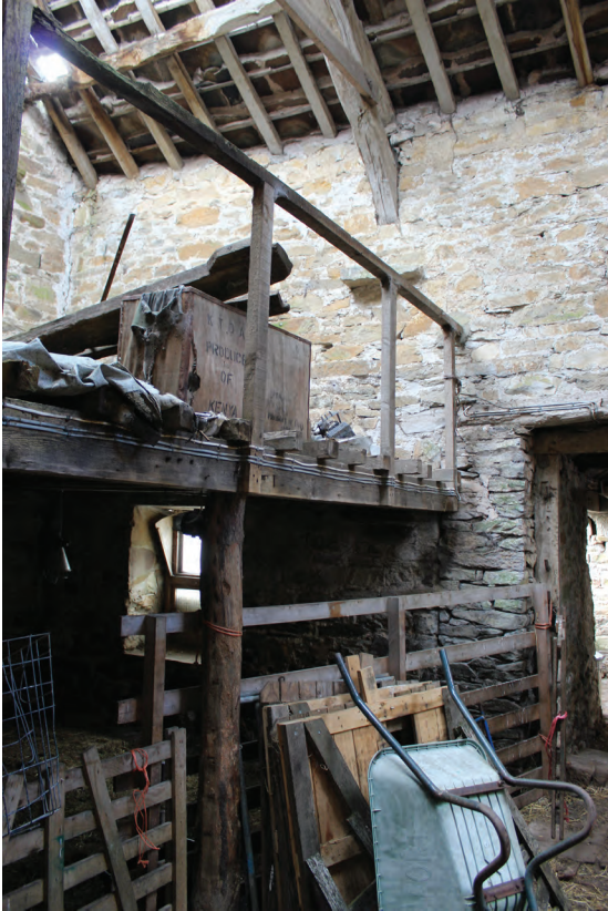
Figure 27 Southern extent of west wall of Room G2, facing south-west. Scale 1x2 m
