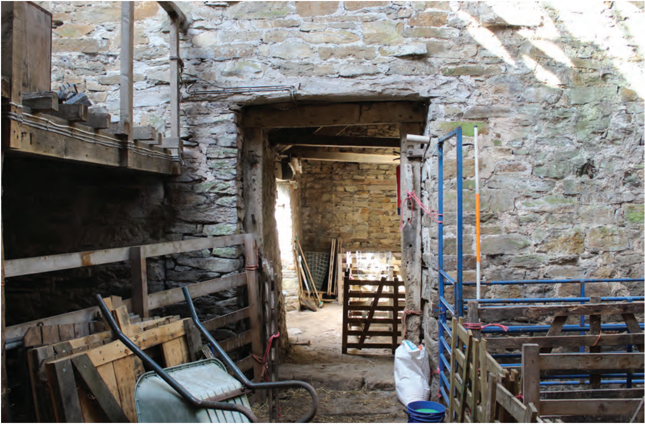
Figure 26 Central section of west wall of Room G2, facing west. Scale 1x2 m
