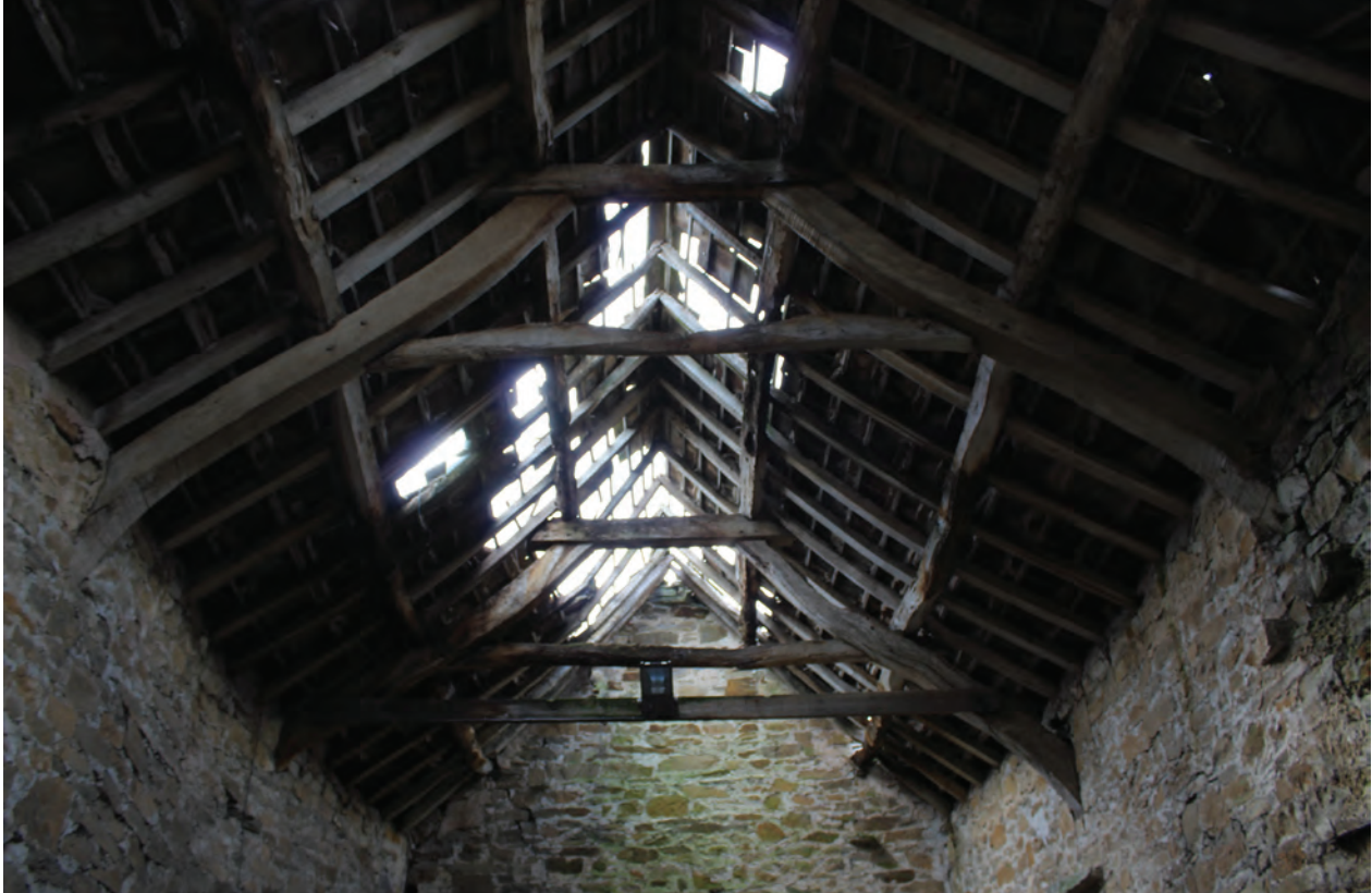
Figure 29 Detail of southern extent of roof structure in Room G2, looking south. No scale
