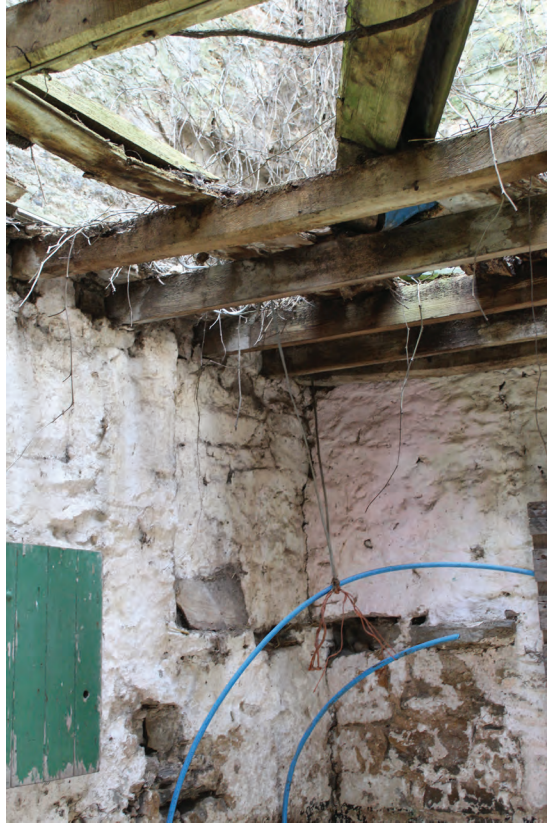
Figure 11 Detail of blocked doorway in south-west corner of Room LG1, facing south-west. No scale
