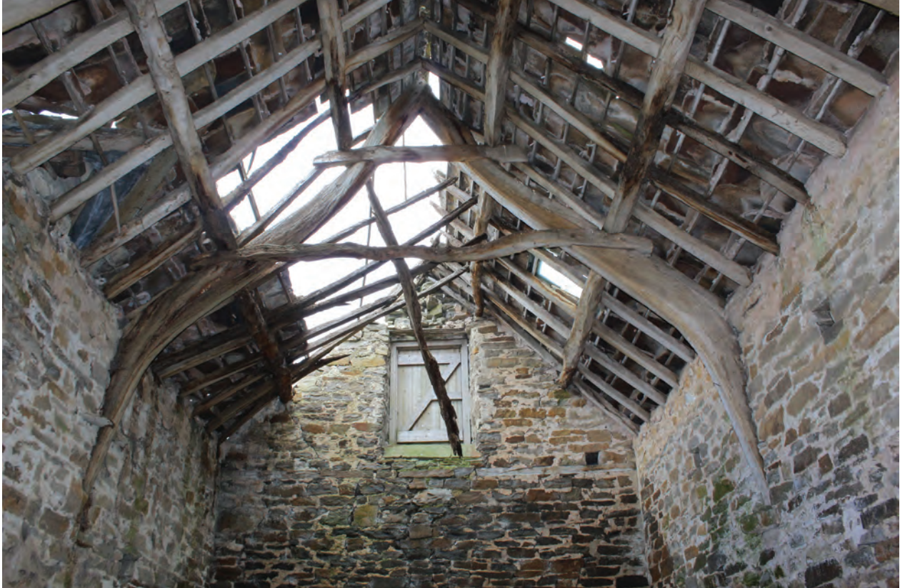
Figure 28 Detail of northern section of roof structure in Room G2, facing north. No scale
