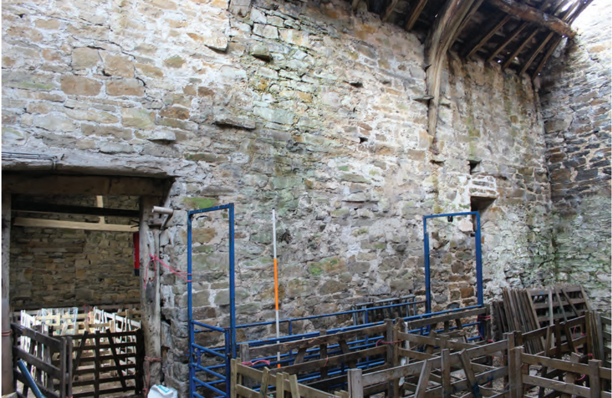
Figure 25 Northern extent of west wall of Room G2, facing north-west. Scale 1x2 m
