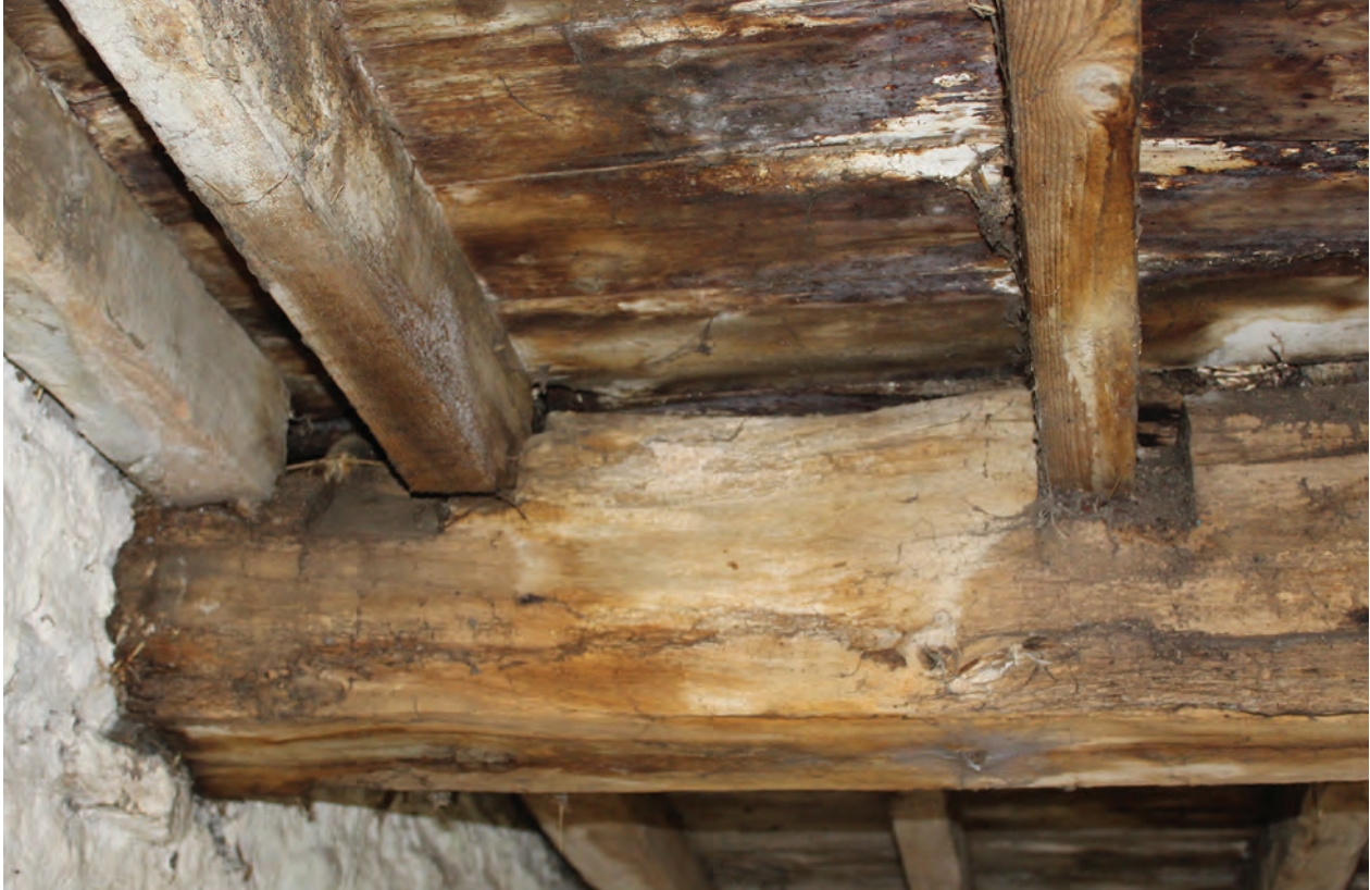
Figure 12 Detail of angled sockets for staircase strings in southern face of principal floor joist, facing north-west. No scale
