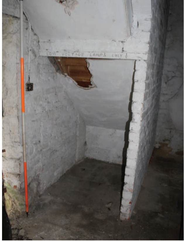
Figure 159 View of inserted stair with blocked door in north wall behind, facing north-east. No scale
