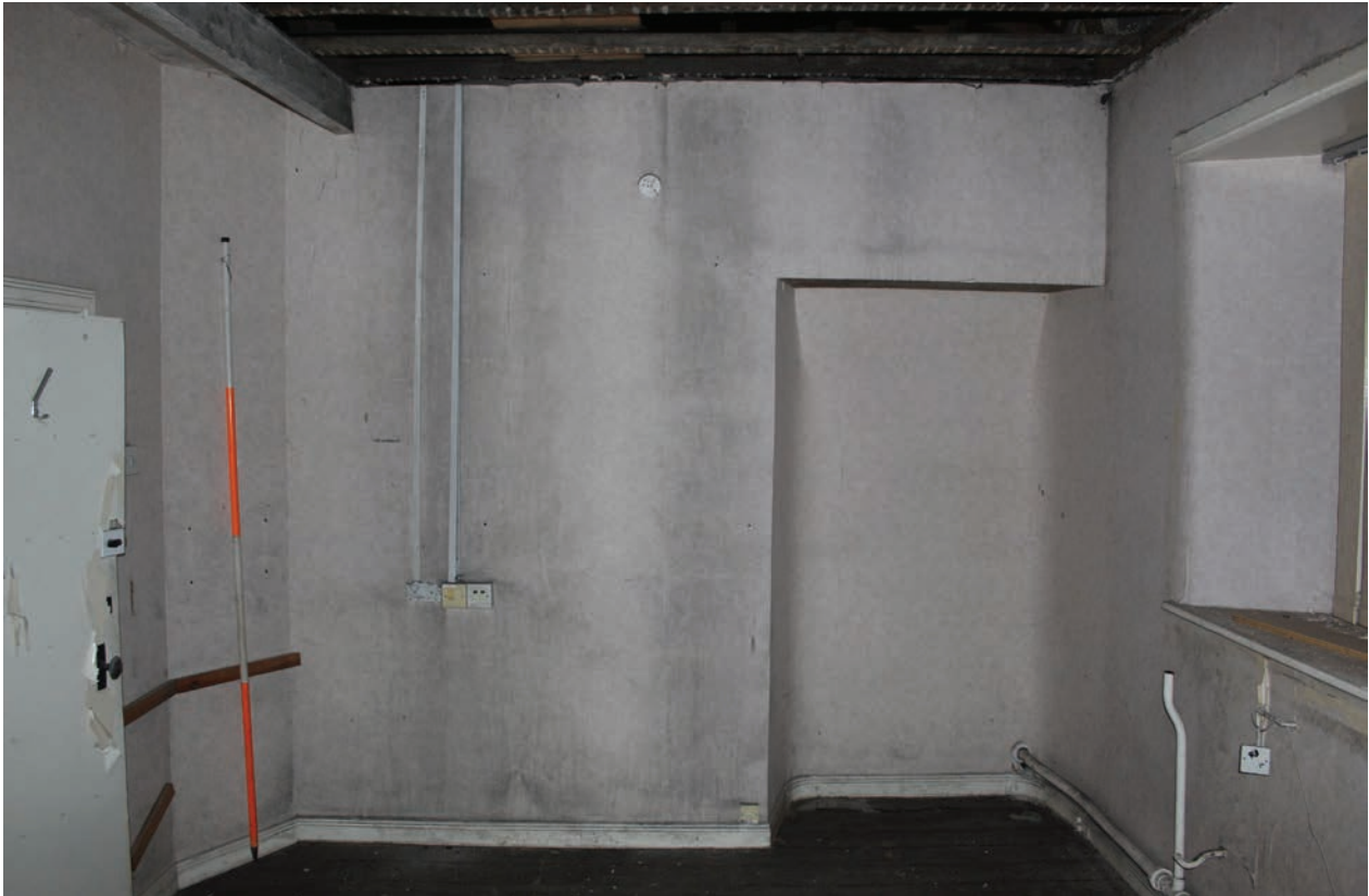
Figure 79 East wall of Room F26, facing east. Note blocked doorway to right. Scale 1x2 m
