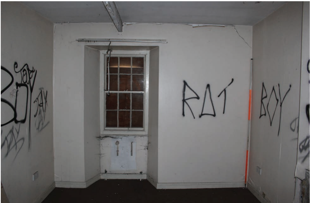
Figure 171 North wall of Room F12 showing window matching that in the south wall of this room and in Room F13. Scale 1x2 m
