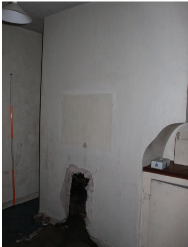
Figure 151 Room G26, facing south-west. Note break in modern plasterboard to examine blocked fireplace. Scale 1x2 m
