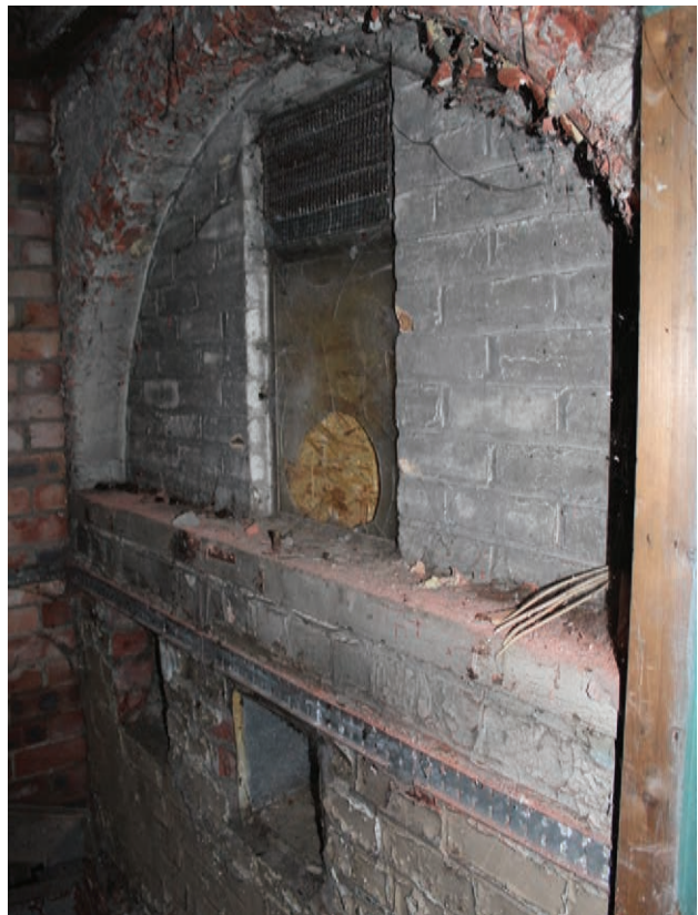
Figure 137 The blocked arch in the north wall of Room G15a, facing north-west. No scale
