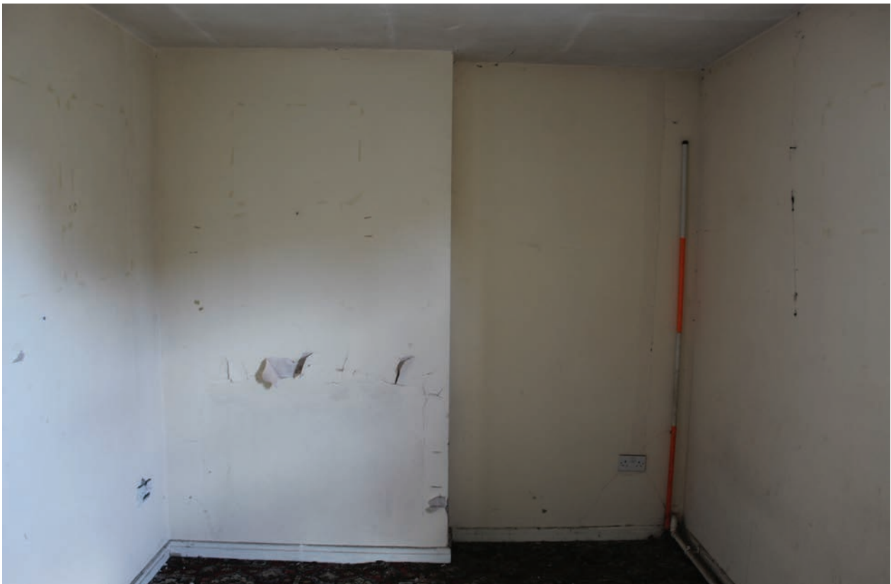
Figure 181 North wall of Room F25. Note blocked fireplace to left. Scale 1x2 m
