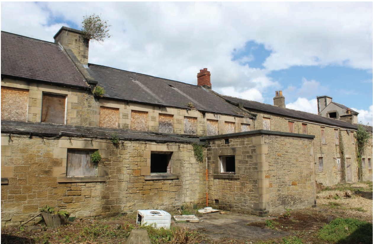
Figure 92 Detail of ranges with clerestory glazing in the 1883 portion of the south elevation of Building B, facing north-east. Scale 1x2 m
