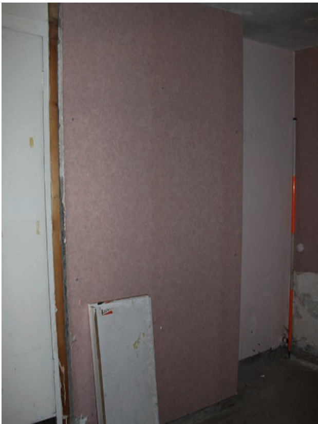
Figure 42 East wall of Room G30, facing south-east. Note the angled stud walling to create deep cupboard space in each of the two rooms. Scale 1x2 m
