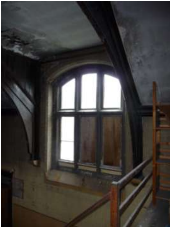
Plate 18. Two of the most significant architectural features are the roof timbers springing from corbels and the mullioned and transomed windows
