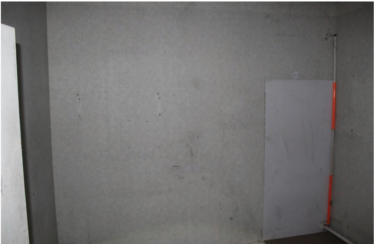
Figure 83 East wall of Room F35, facing east. Note blocked doorway to right. Scale 1x2 m
