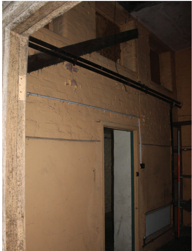
Figure 139 Room G15, facing north-west and showing doorway and clerestory windows. Scale 1x2 m
