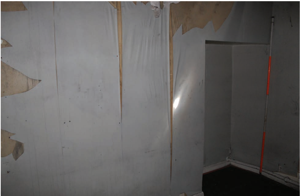
Figure 76 East wall of Room F25, facing south-east. Note blocked doorway at right. Scale 1x2 m
