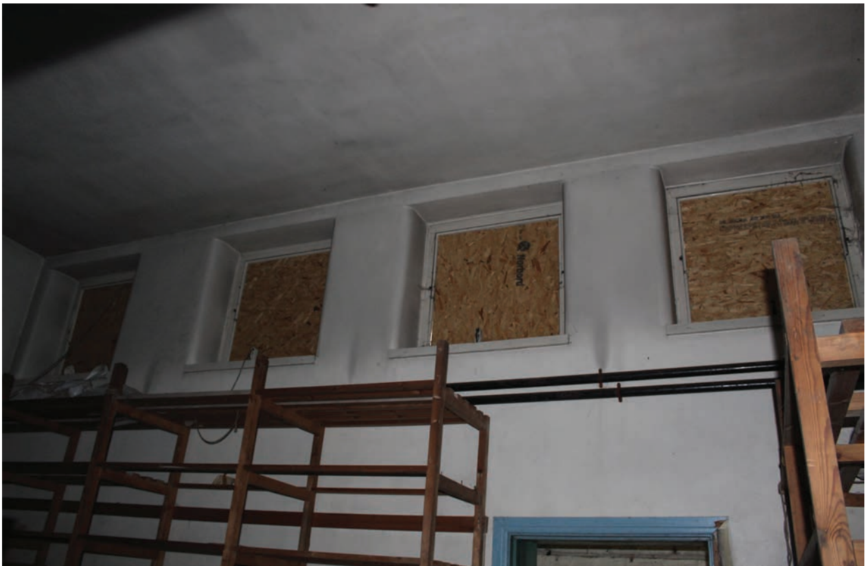
Figure 141 Detail of clerestory windows in north wall of Room G19, facing north. No scale
