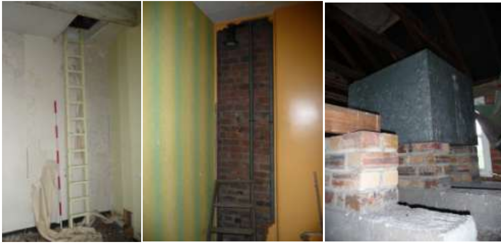
Plate 28. The ladder to the water tank in room 88 (left) and the pipes on the walls in room 87 (right). The water tank appears to be of lead and is supported on concrete beams and brick pillars.
