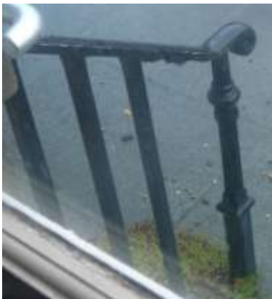
Plate 33. At the top of the stairs (FC101) is a 1930s half glazed doorway with Victorian three pane overlight which affords access to external flat roof space (over FC 19 and 20) - the presence of wrought iron balustrades suggest that this was a fire escape designed by Morton and typical of the late 19 th century responses to tragic deaths in workhouses elsewhere
