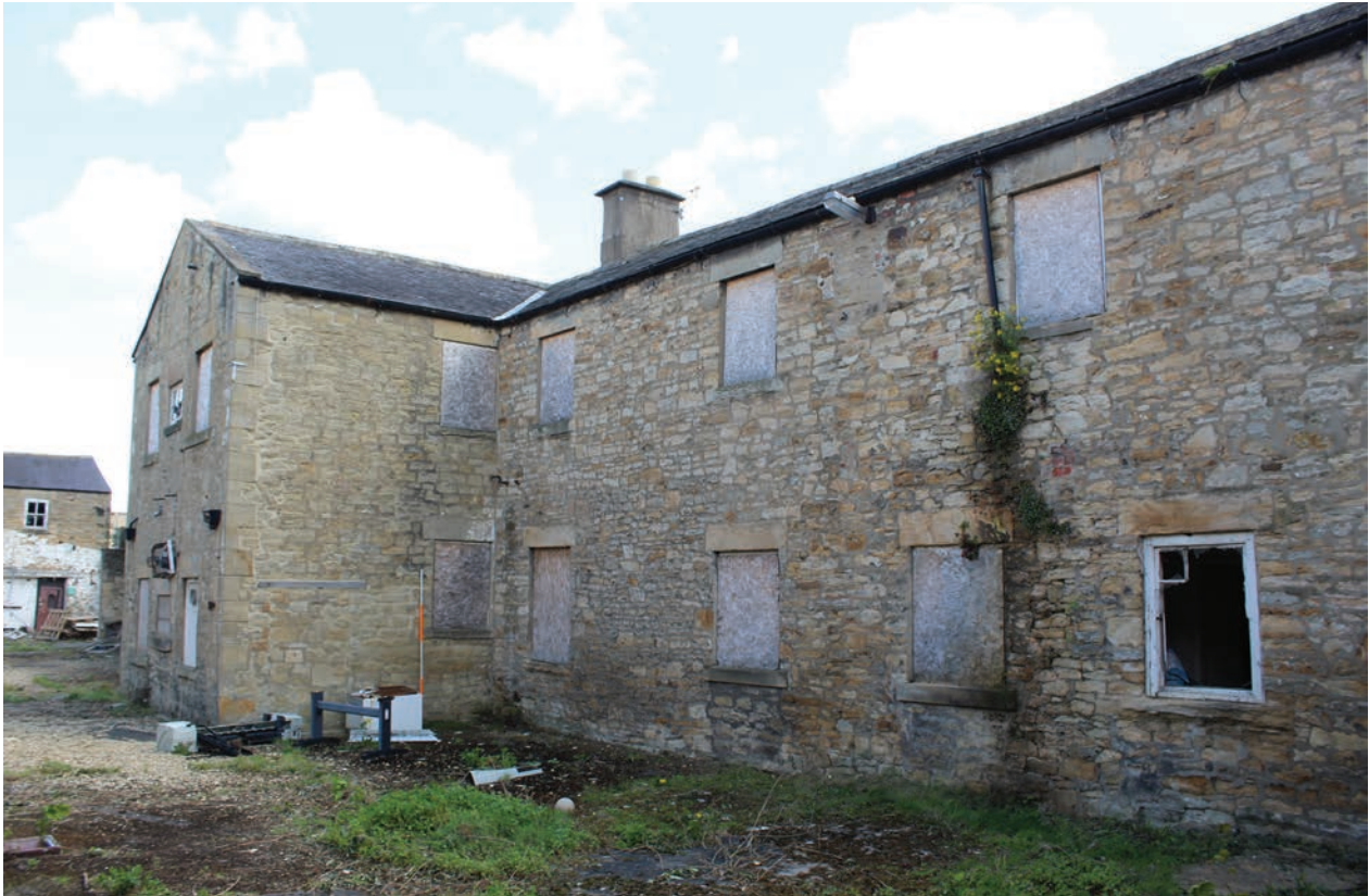
Figure 12 Eastern end of north elevation of Building A, facing south-east. Scale 1x2 m
