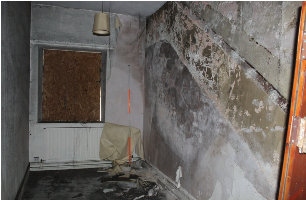
Figure 117 Room G2, looking north-east. Note scar of former staircase on east wall. Scale 1x2 m
