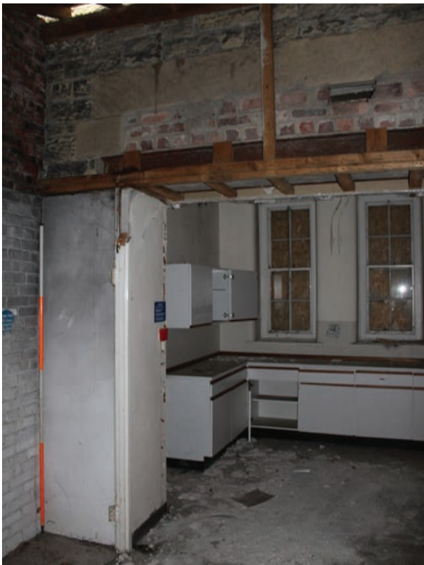
Figure 213 North wall of Room G2, facing north-west. Note former window lintel above inserted opening. Scale 1x2
