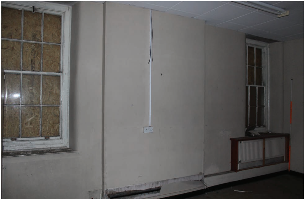
Figure 215 North wall of Room G3 showing location of original fireplace between the windows. Scale 1x2 m
