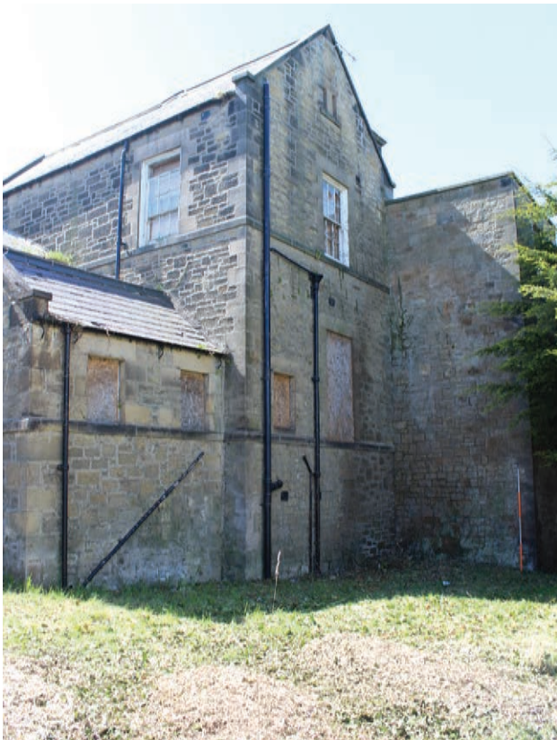
Figure 203 Detail of the north elevation of the projecting bay of the 1883 extension to the north elevation of Building C, facing south-west. Scale 1x2 m
