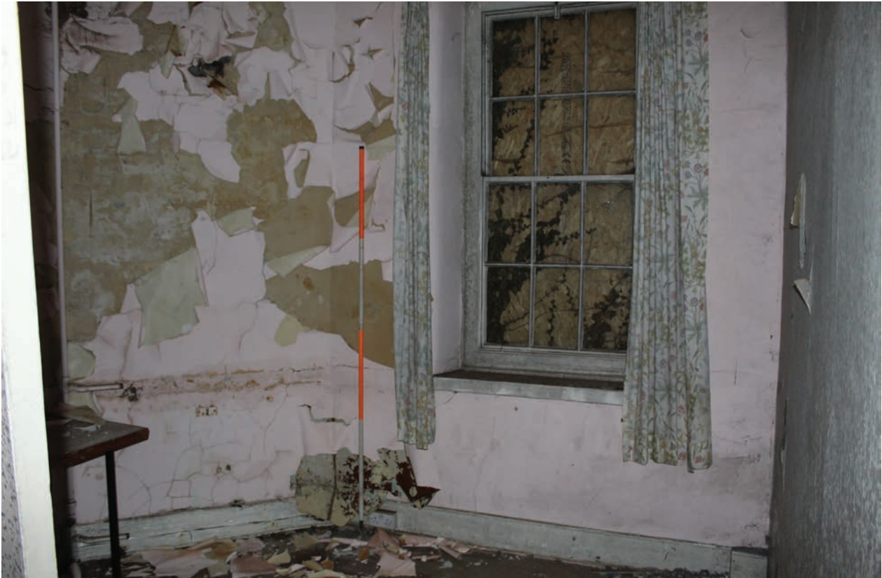
Figure 219 Facing north-west in Room G11, showing original window and angled wall concealing blocked fireplace. Scale 1 x 2 m
