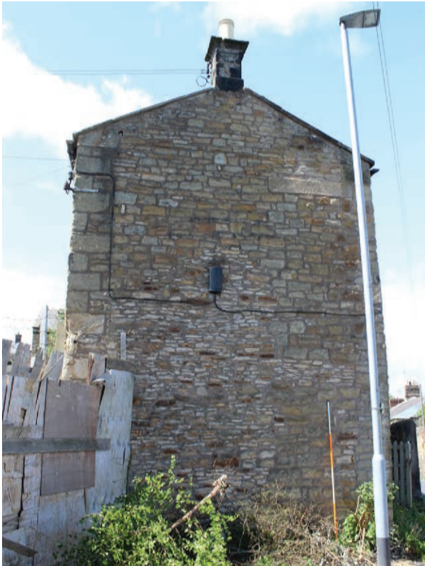
Figure 207 Detail of the north elevation of the projecting bay of the 1883 extension to the north elevation of Building C, facing south-west. Scale 1x2 m
