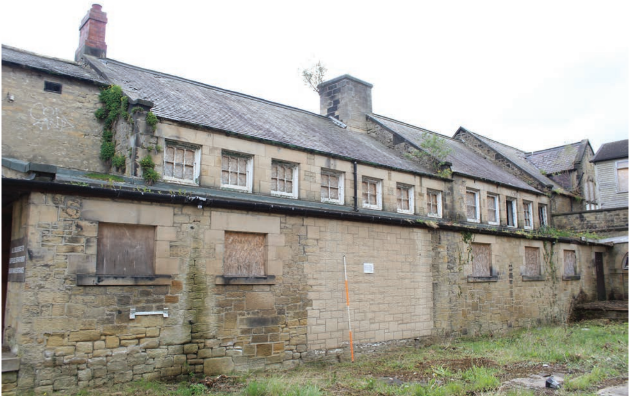
Figure 106 Detail of ranges with clerestory glazing in the 1883 portion of the north elevation of Building B, facing south-east. Scale 1x2 m
