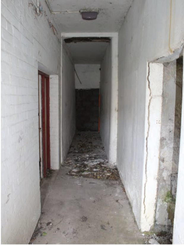
Figure 158 Room G37, facing east. Note blocked door to right and two phases of construction in north wall to left. Scale 1x2 m
