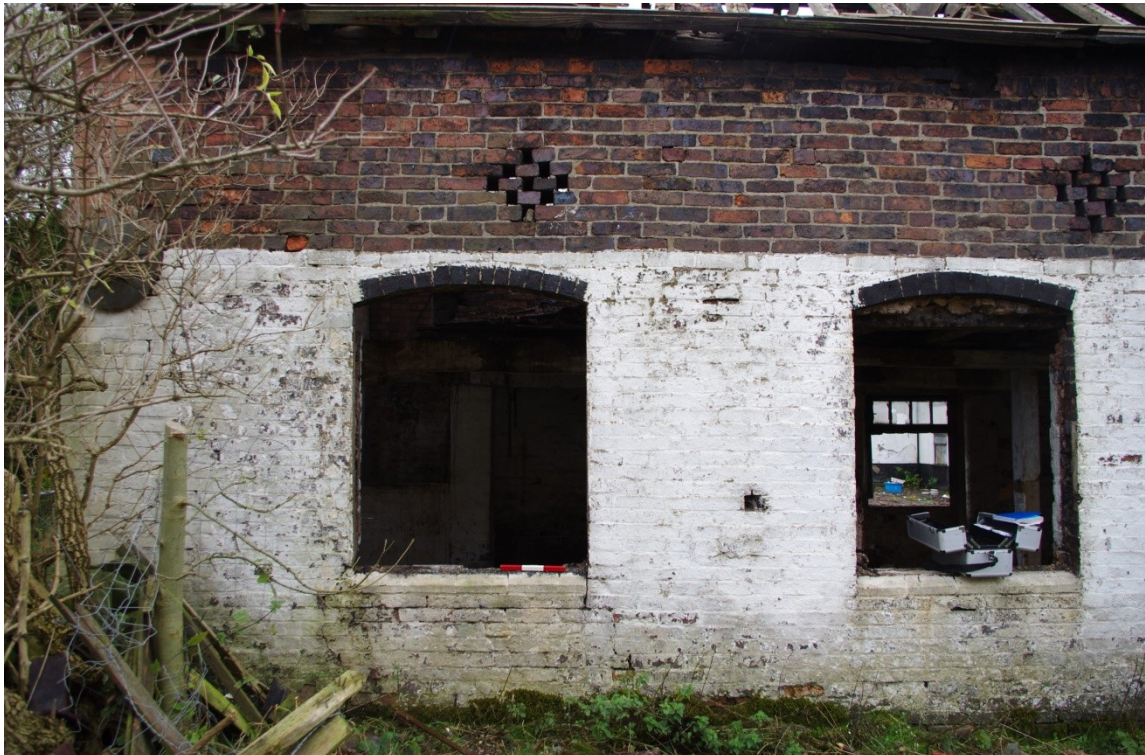
Figure 10 Straight Joint & Partially Blocked Door at North Eastern End of Rear Elevation.
