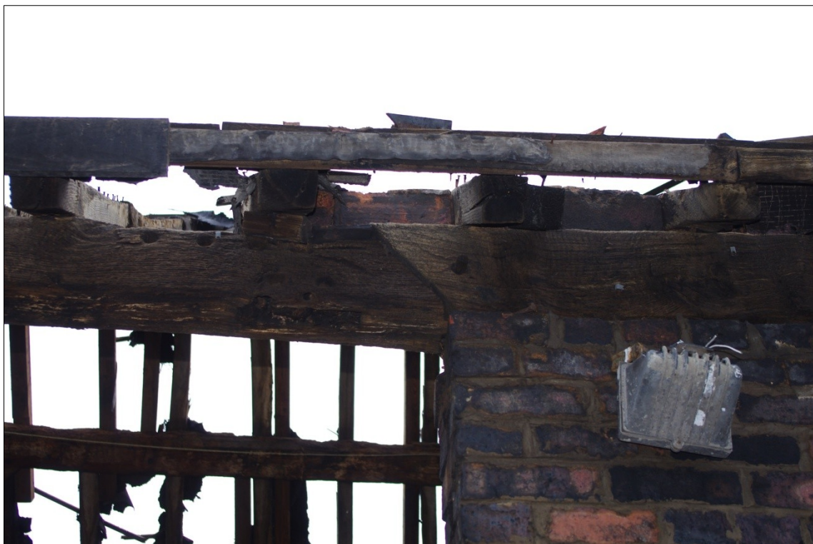
Figure 15 Scarfed Joint & Empty Peg Holes on Principal Elevation Wall Plate.
