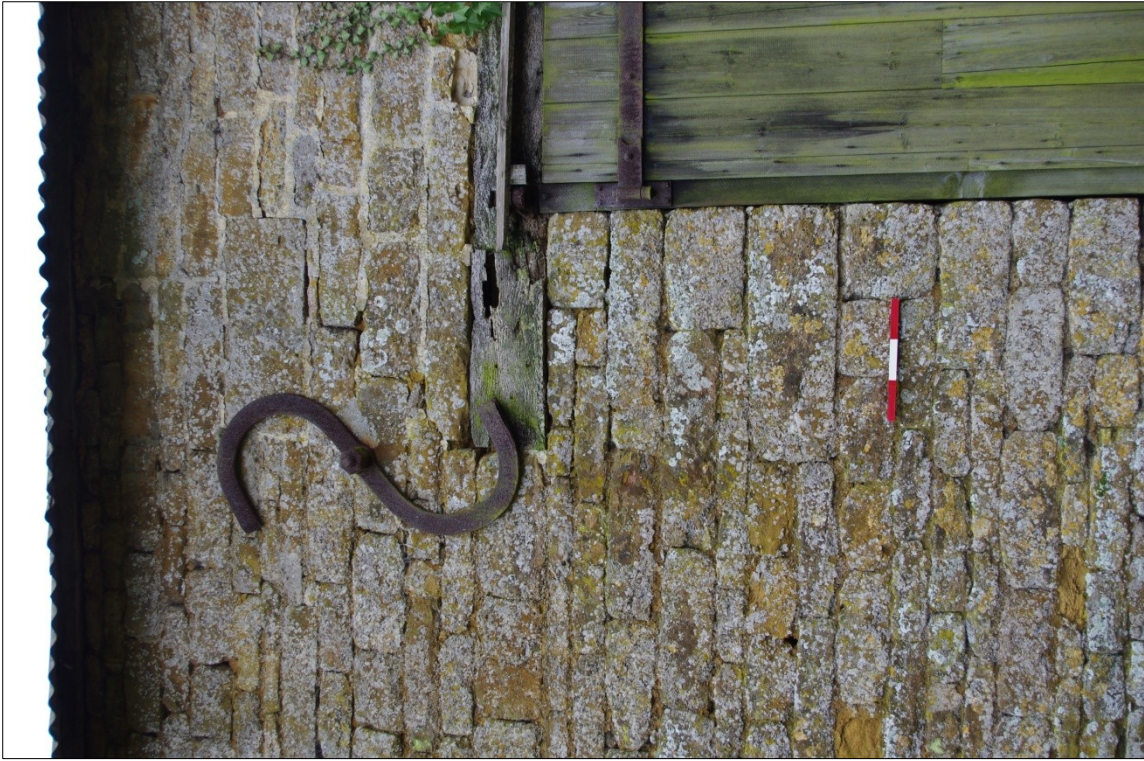
Figure 11 Straight Joint Visible Above Rear Door of A .
