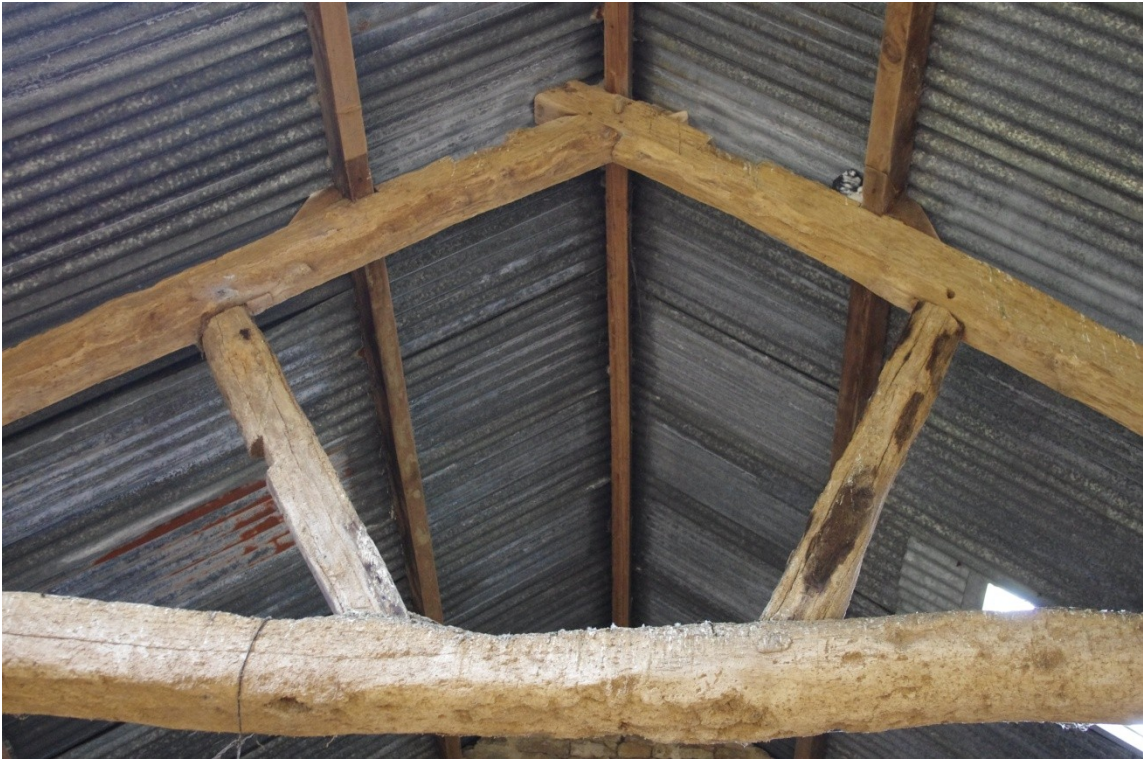
Figure 15 Truss Tr04 Showing Potentially Altered Mortice Holding Left Strut and Higher Open Trenches for Purlin.
