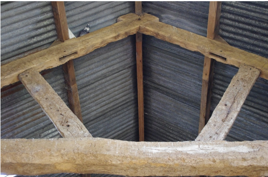
Figure 16 Truss Tr01 Showing Inscribed Assembly Marks and Open Mortices.
