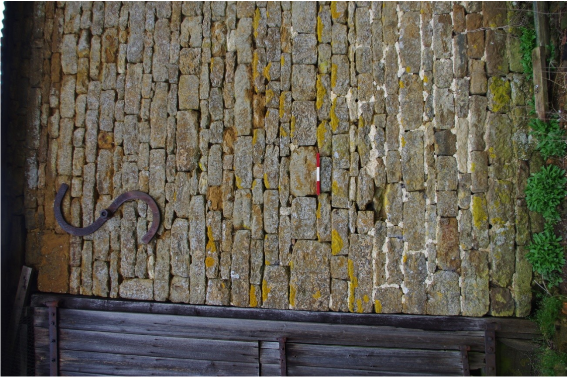
Figure 9 Banding Visible on Principal Elevation of B .
