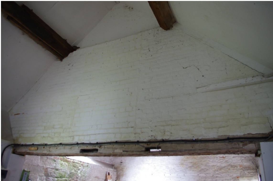
Figure 17 Brick-Built Wall & Blocked Opening Carried on Tie Beam in D (looking South West).
