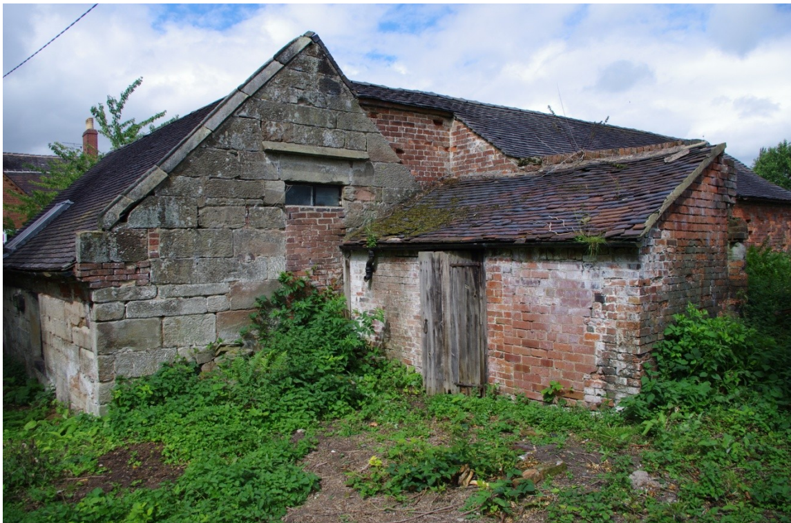
Figure 11 East Facing Gable D (left) and Principal Elevation E (looking West – North West).
