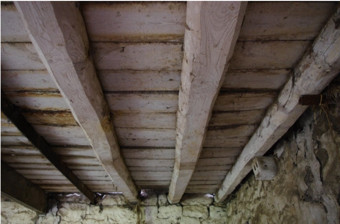
Figure 20 Building 02A, Flattened Joists.
