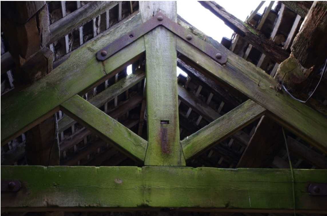
Figure 22 Building 02A Open Mortise on Underside of Purlins Indicating Position of Original Truss.
