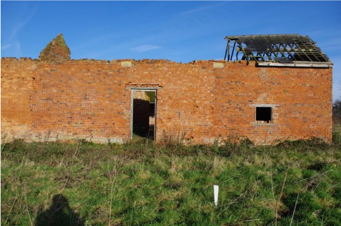
Figure 10 Building E South Facing Elevation Showing Blocked Threshing/Cart Door (looking North East).
