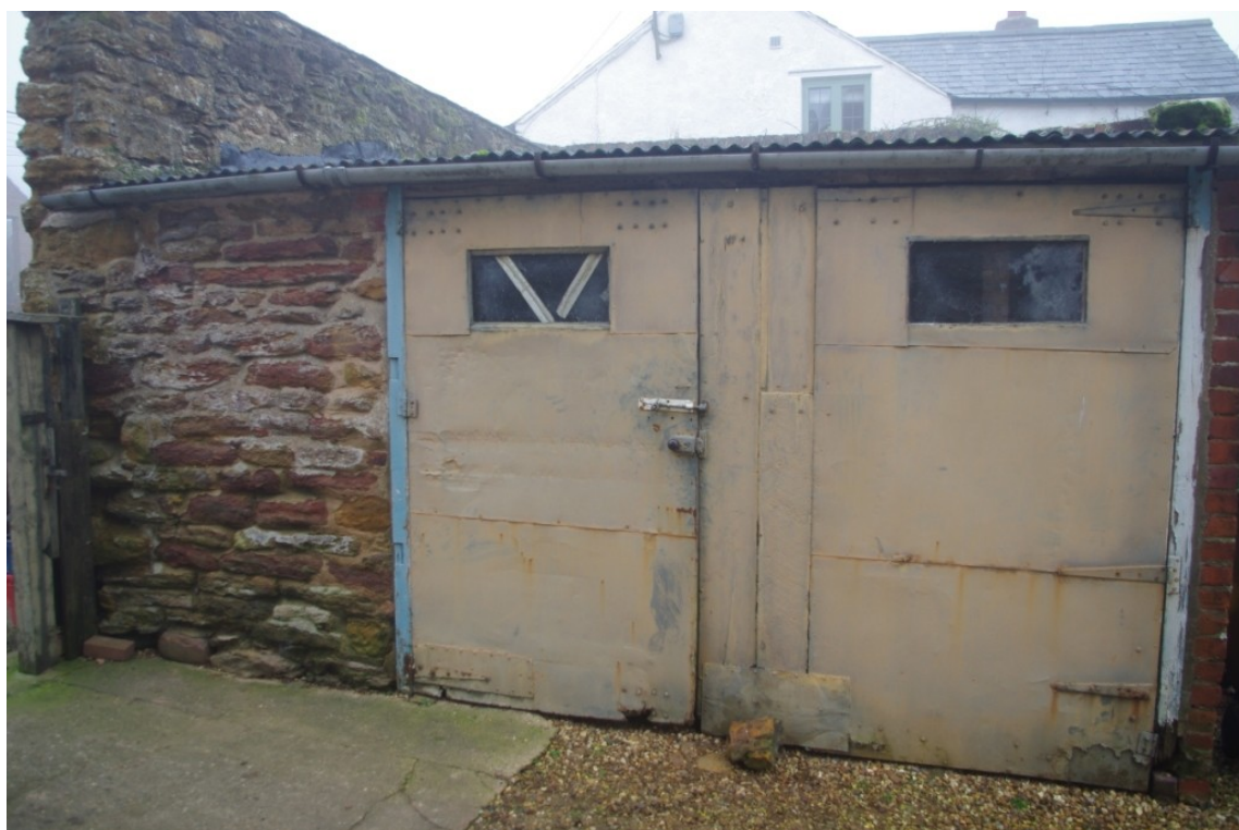
Figure 9 Building A North Facing Elevation Showing Door & Fire Reddened Stones (Left).
