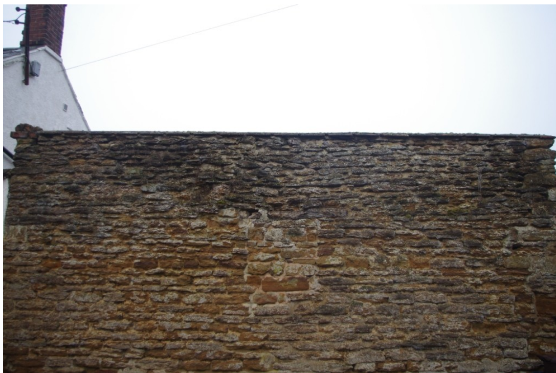
Figure 8 Building A Harbidges Lane Elevation Showing Replaced Upper Courses & Blocked Window.
