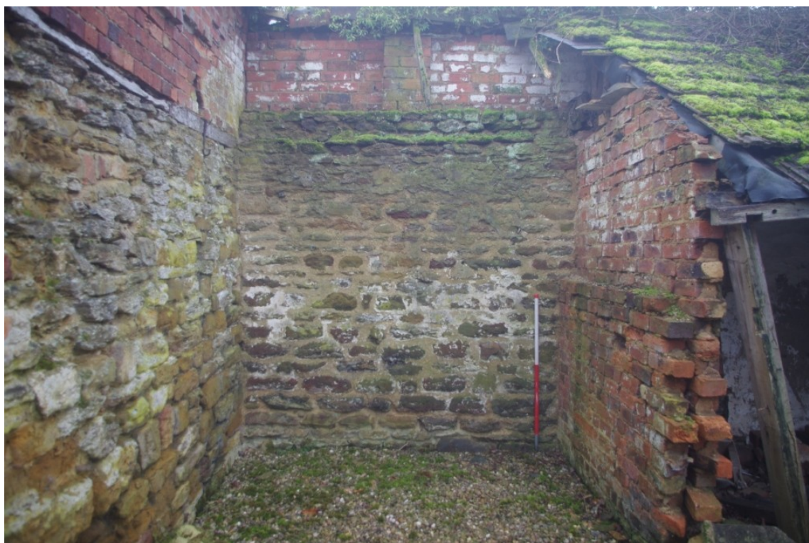
Figure 16 Boundary Wall Showing Upper Brick Courses.
