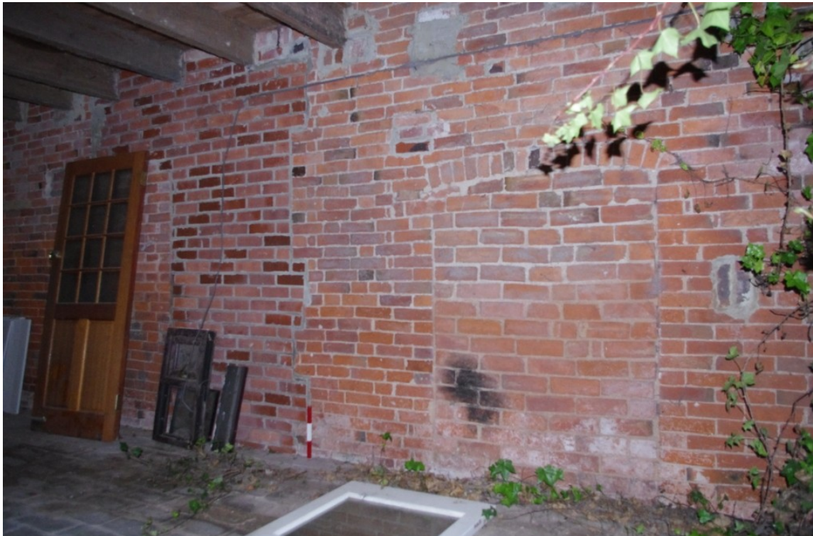
Figure 10 Building A (3) Blocked Openings in West Facing Wall.
