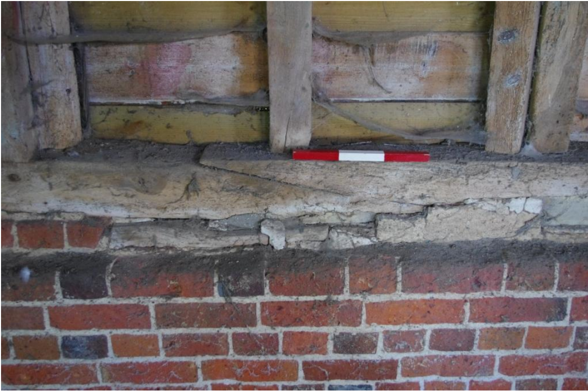
Figure 13 Scare Joint on Sill Beam, Internal View.
