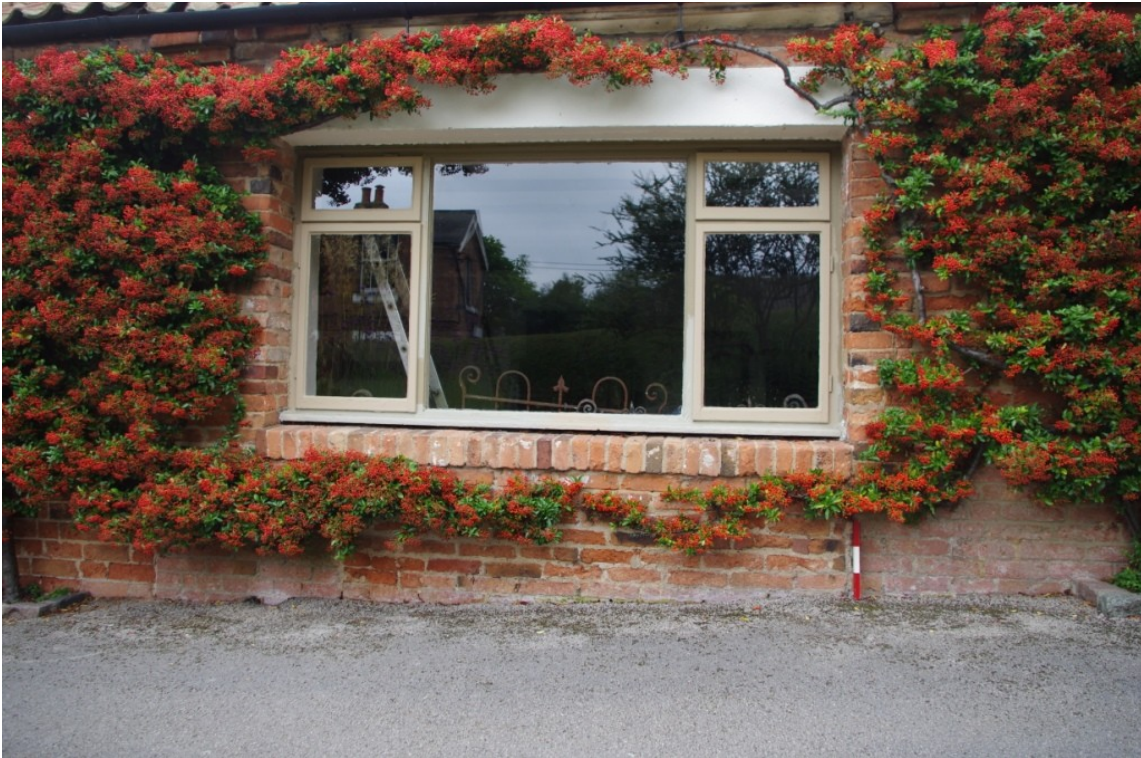
Figure 9 Building A (1) Possible Blocked Opening on Principal Elevation Visible Below Inserted Window.
