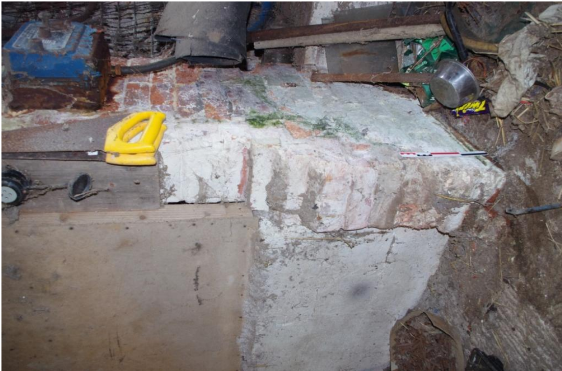
Figure 9 Remnant of Sleeper Wall on Principal Elevation, Internal (Looking East - South East).
