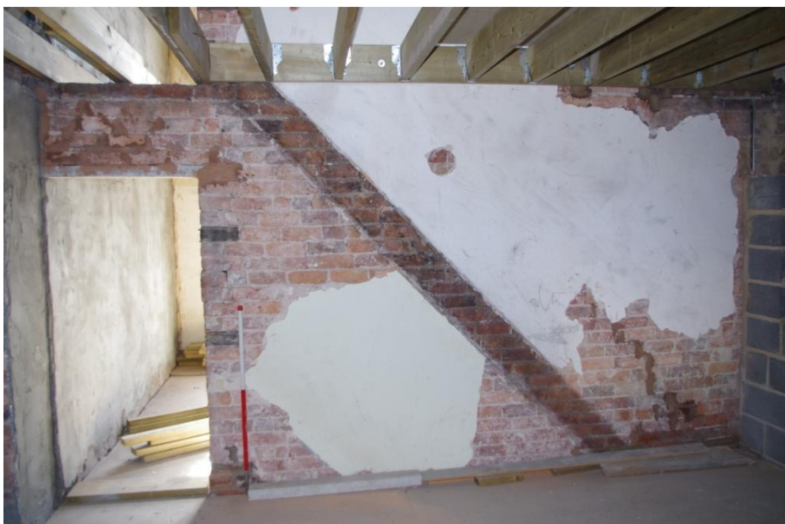
Figure 10 A (05) Outline of Stair Stringer on West – North West Facing Wall (Looking East – South East).
