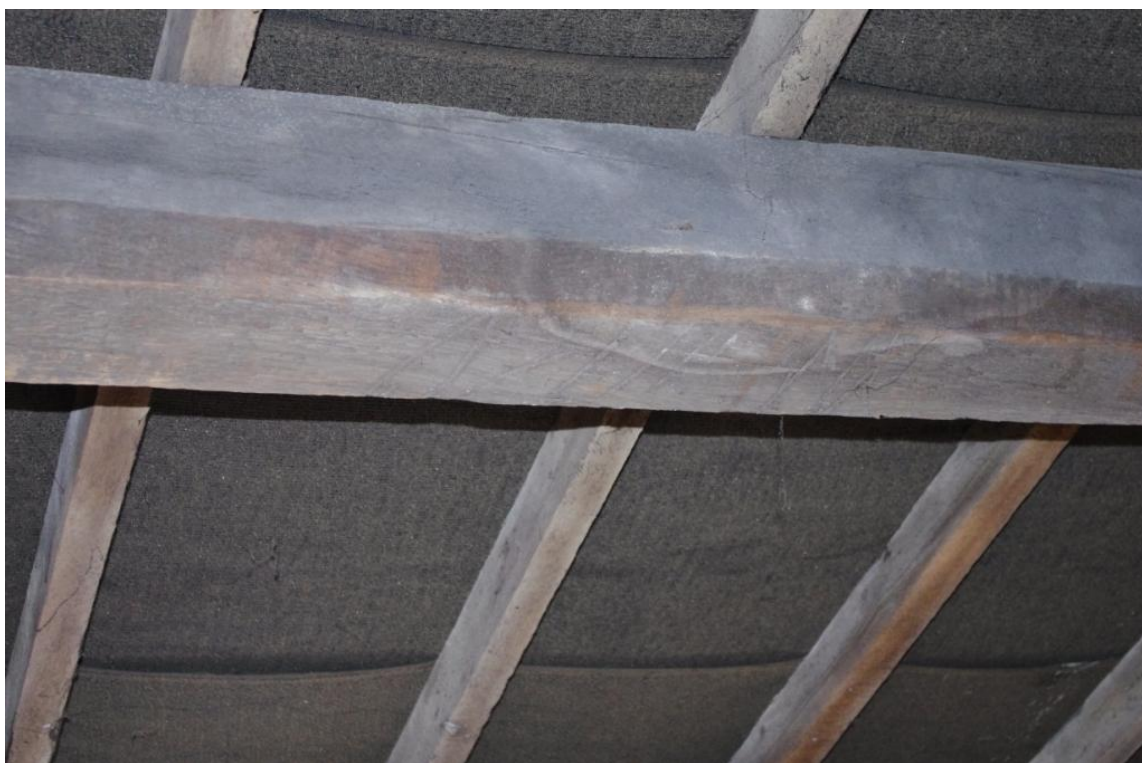
Figure 17 B(07) Rase Marked Purlin.
