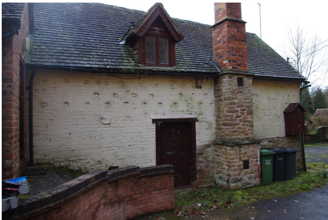
Figure 16 The Lodge, Rear Elevation Showing Modern Chimney & Missing Brick Ventilation (Looking South West).
