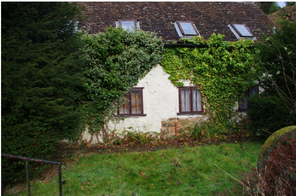
Figure 13 The Lodge, Principal Elevation, Showing Straight Joint in Brickwork (Looking North East).
