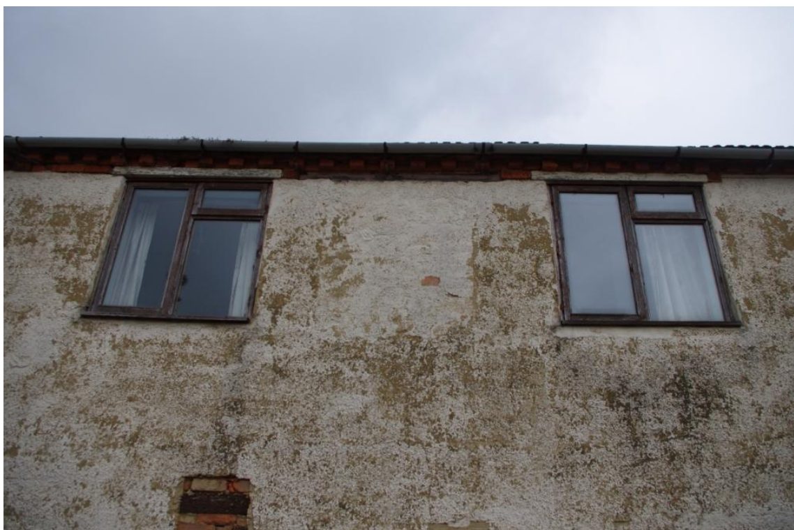
Figure 8 Principal Elevation, Evidence of Blocked Window at First Floor Level.
