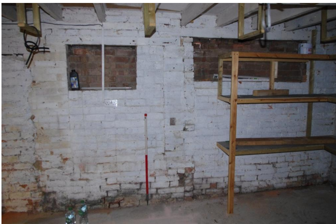
Figure 11 Room (2), Blocked Openings on Principal Elevation, Internal (Looking West – South West).
