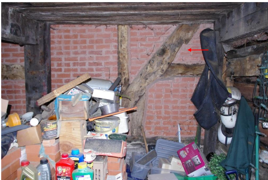
Figure 9 Oblique Tenon Joint (Arrowed) on Angled Brace, Southernmost Gable.
