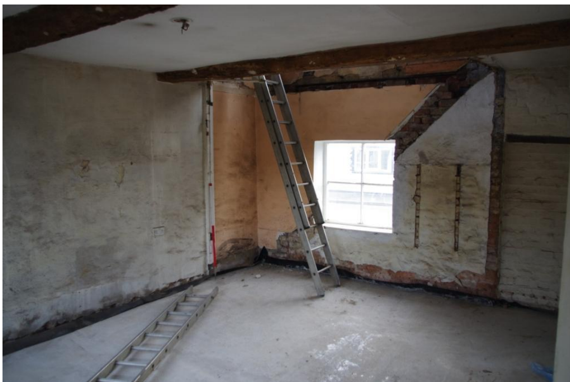
Figure 23 (1), Ghost Stringer Showing Location of Staircase on South Wall (Looking South East).
