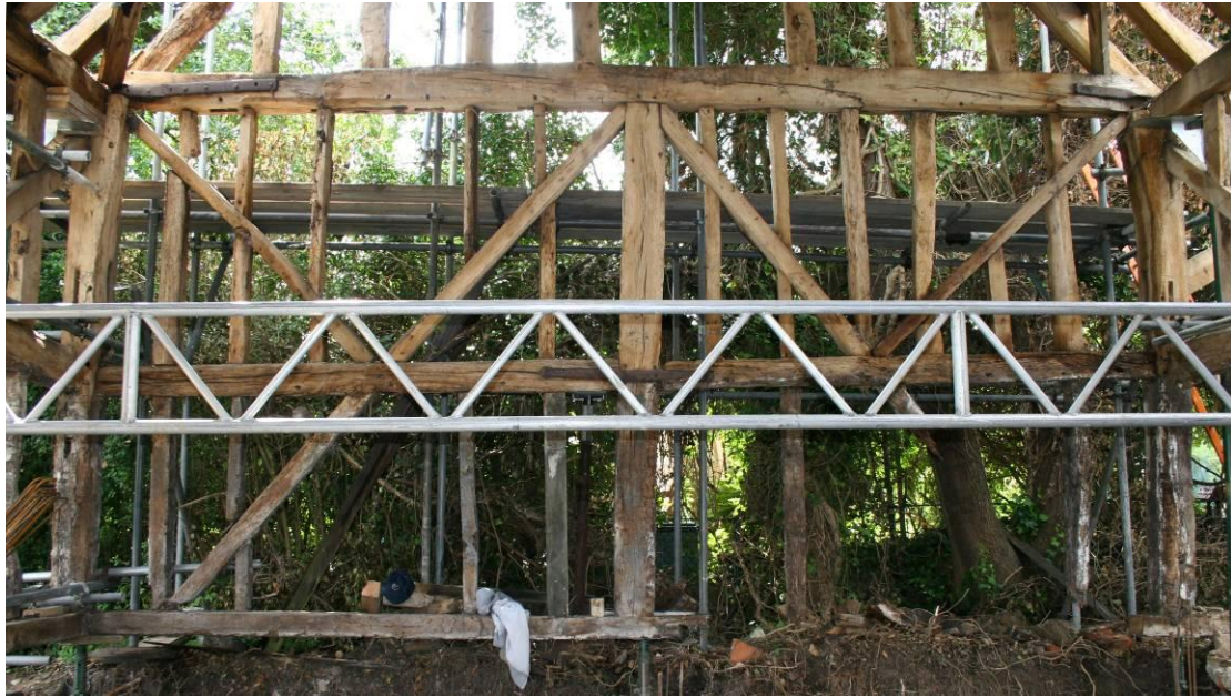
South elevation of the Barn. Note rotted away sole plate.
