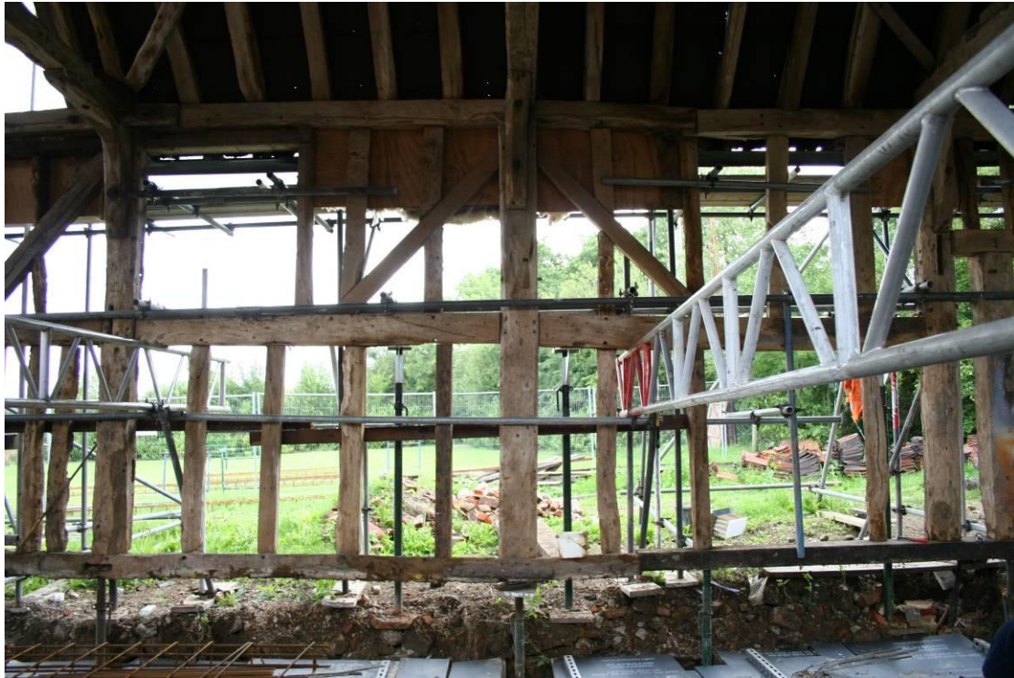
Bays 3 and 4 looking east. Note openings for high level hatch and doorway.
