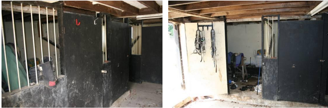
The central bay has been converted into a secure store with loft above. Looking NW and W.
