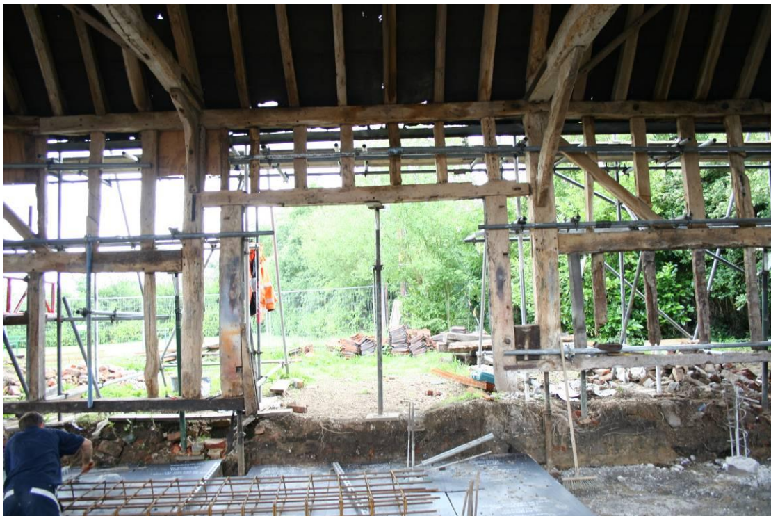
Bay 5. Framed doorway for full height doors. Note hanging knee and straight braces to tie-beams. Also mid-rail removed to insert door lintel.
