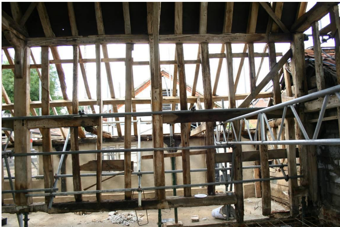
Bays 1 and 2 looking west. Note severed mid-rail and sole plate for former openings.
