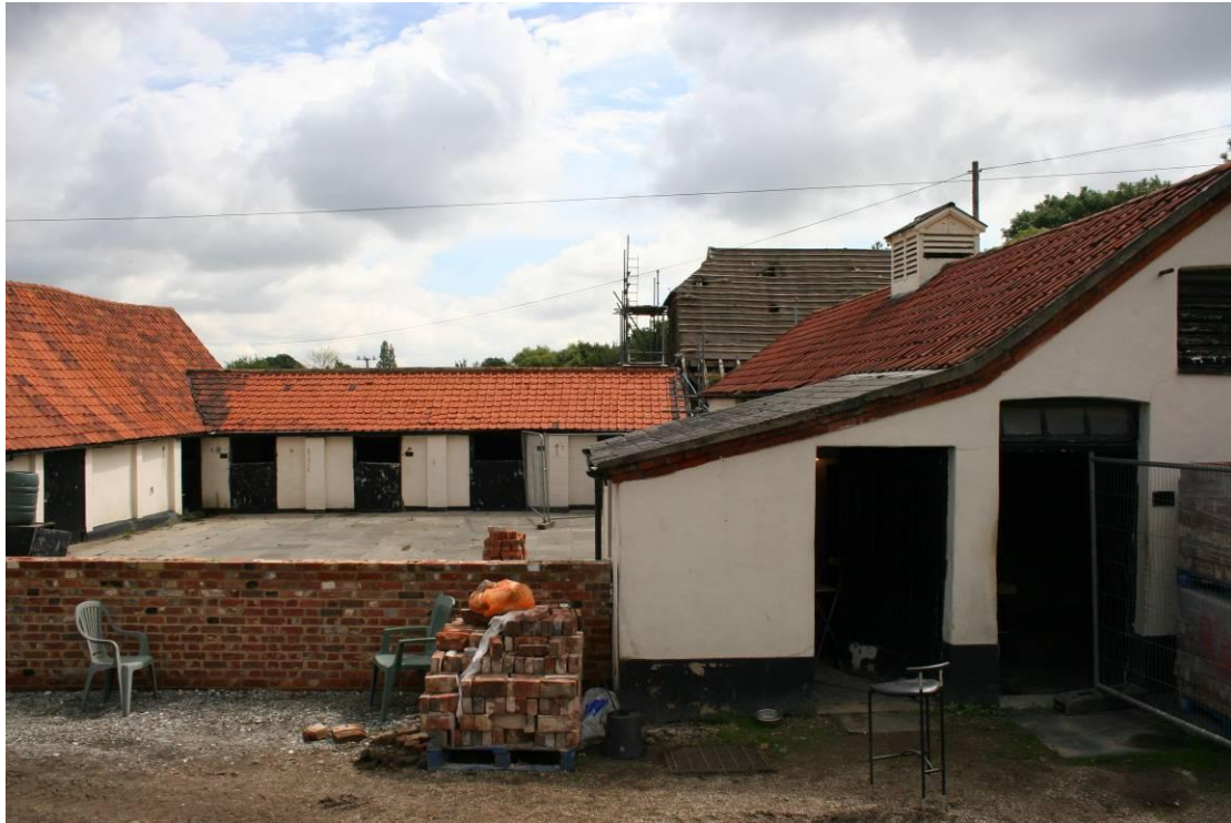
The North, East, Central Stables with Barn roof behind from the west.
