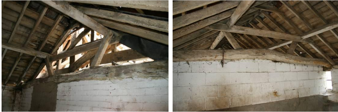
The low-pitch roof has short raking struts to the purlins. Stall 4 looking SE and NE.
