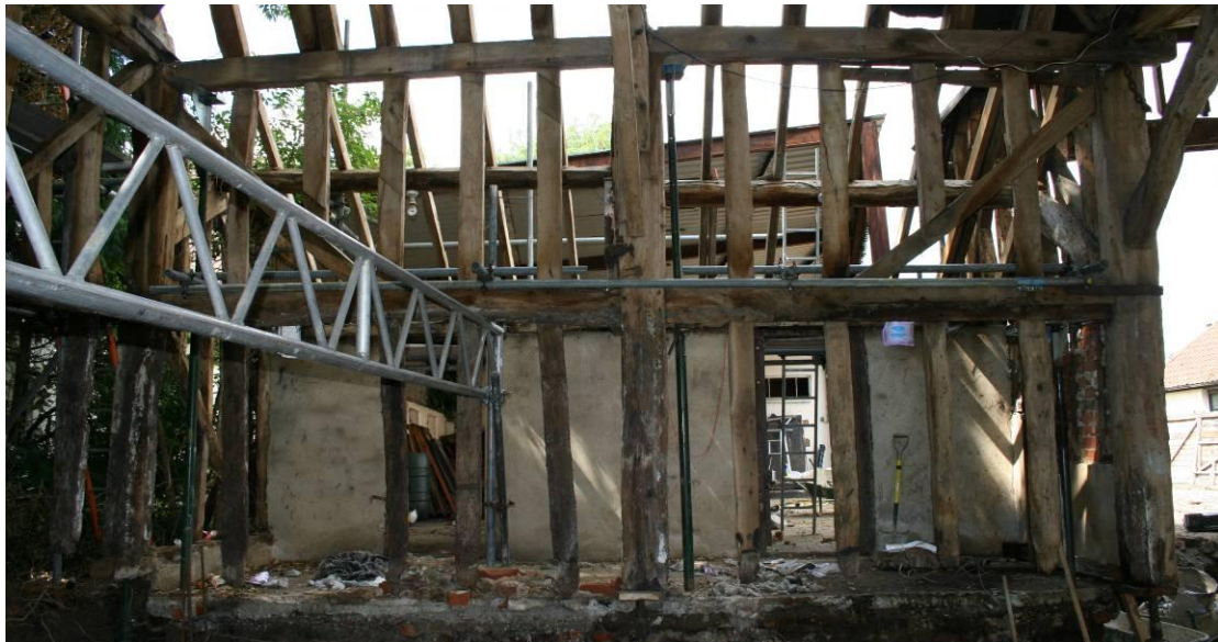
The SW corner of the Barn. Bays 4 and 5. Note trenched studs out of place.
