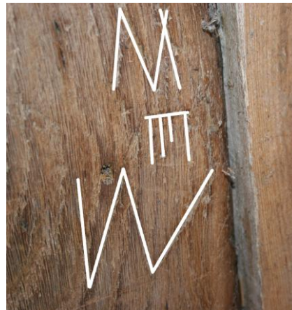
Apotropaic marks on the principal post of Truss 2.
