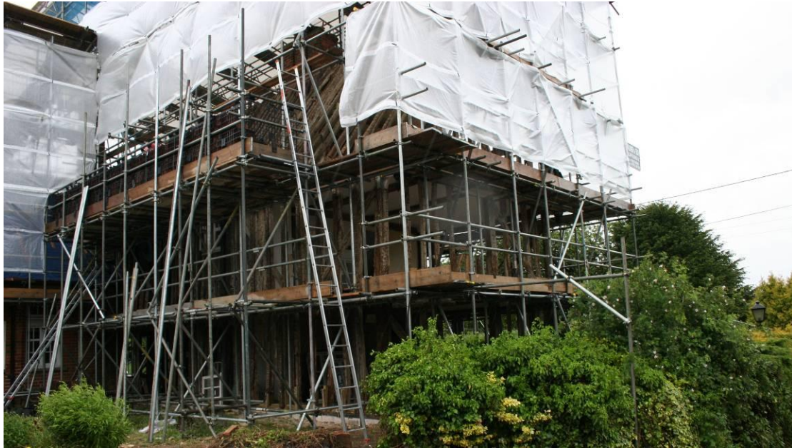
During the strip out the building was clad with protective sheeting. Looking SE.
