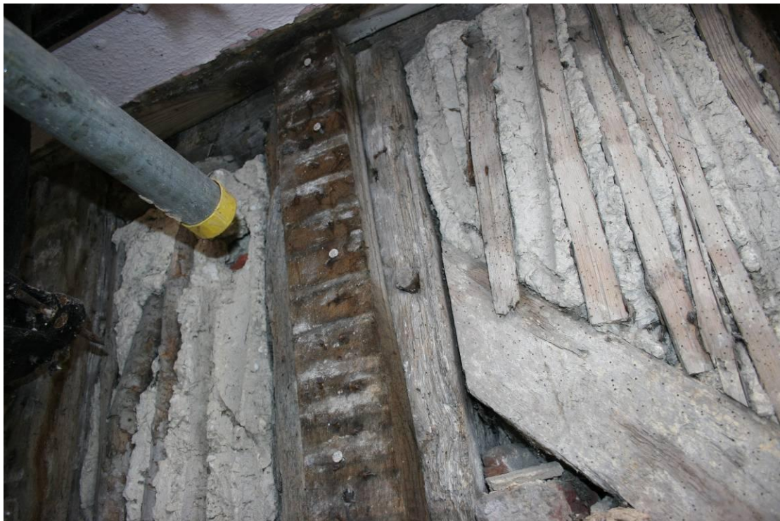
Detail of wattle and daub and lath and plaster panels on the first floor.
