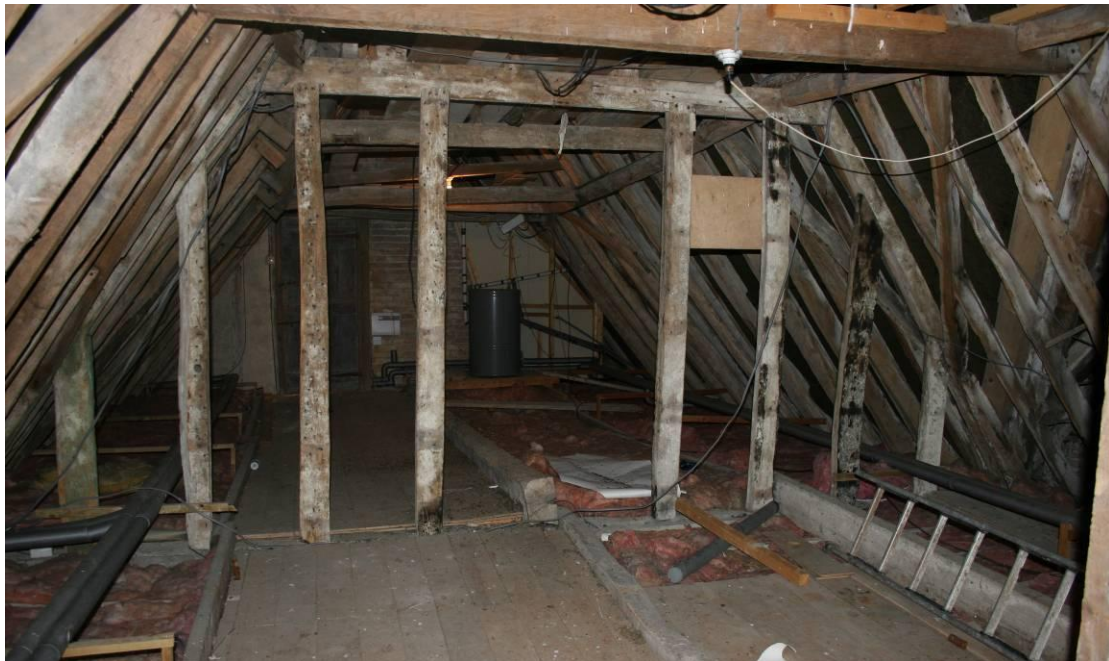
The Eastern Attic was boarded out as two store rooms. Looking W.
