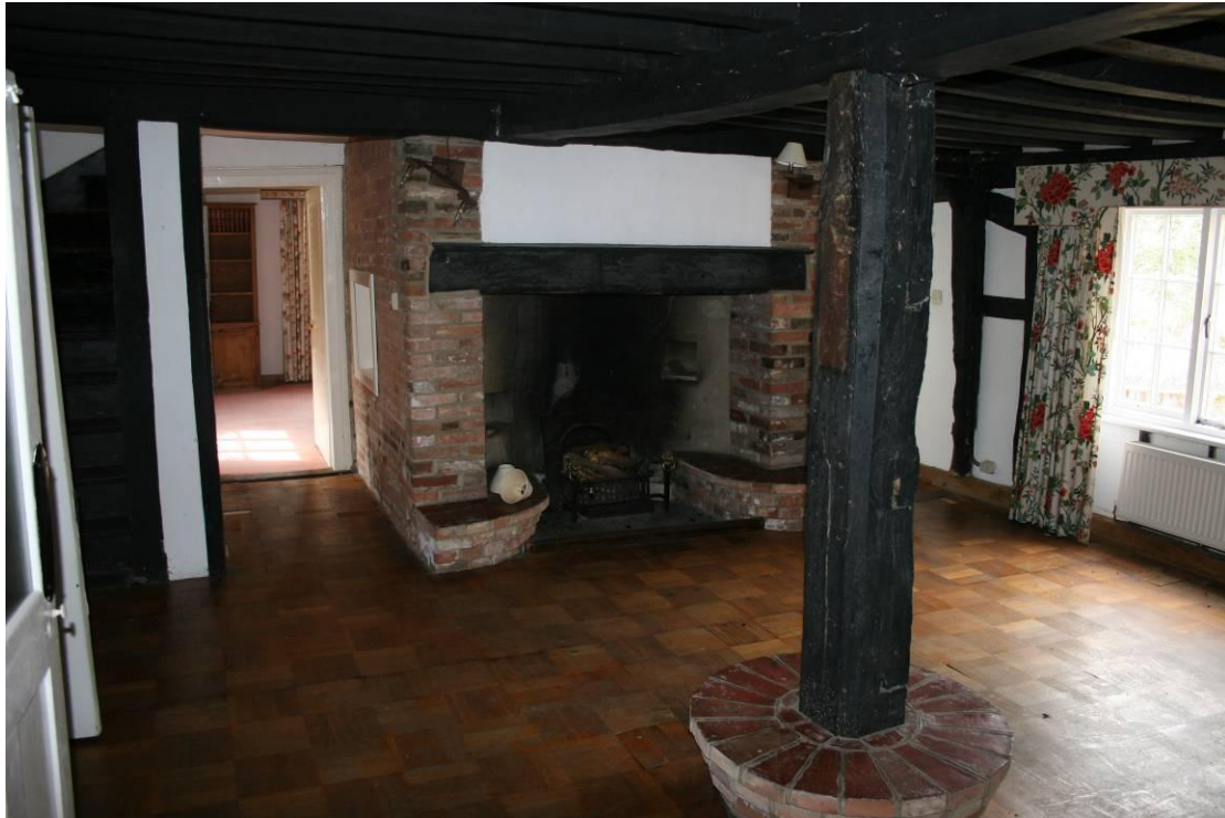
Looking W in the Living Room. The post takes the weight of the failing main joist.
