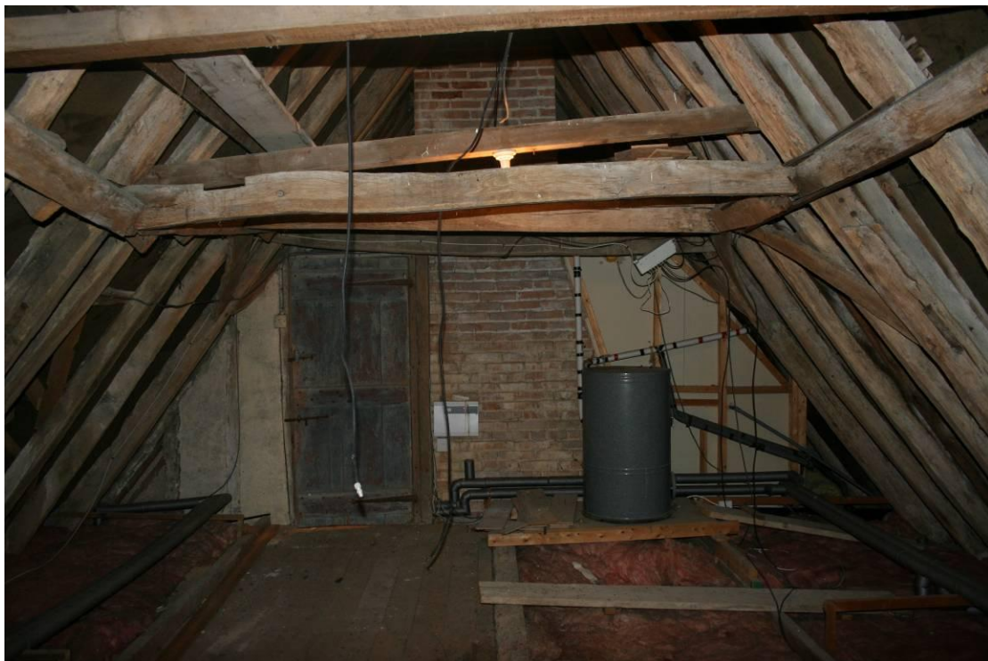
The junction of the original roof with the added eastern roof. Looking W.
