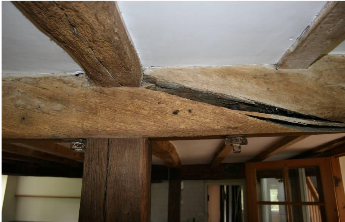
Historic failure addressed with C.1800 style wrought iron bolts.
