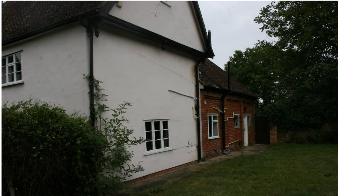
The jettied gable for the attic rooms. The exposed frame is shown below.
