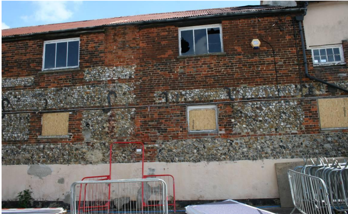
The flint panelling is not consistent. Note the brick patch where the lucam was.
