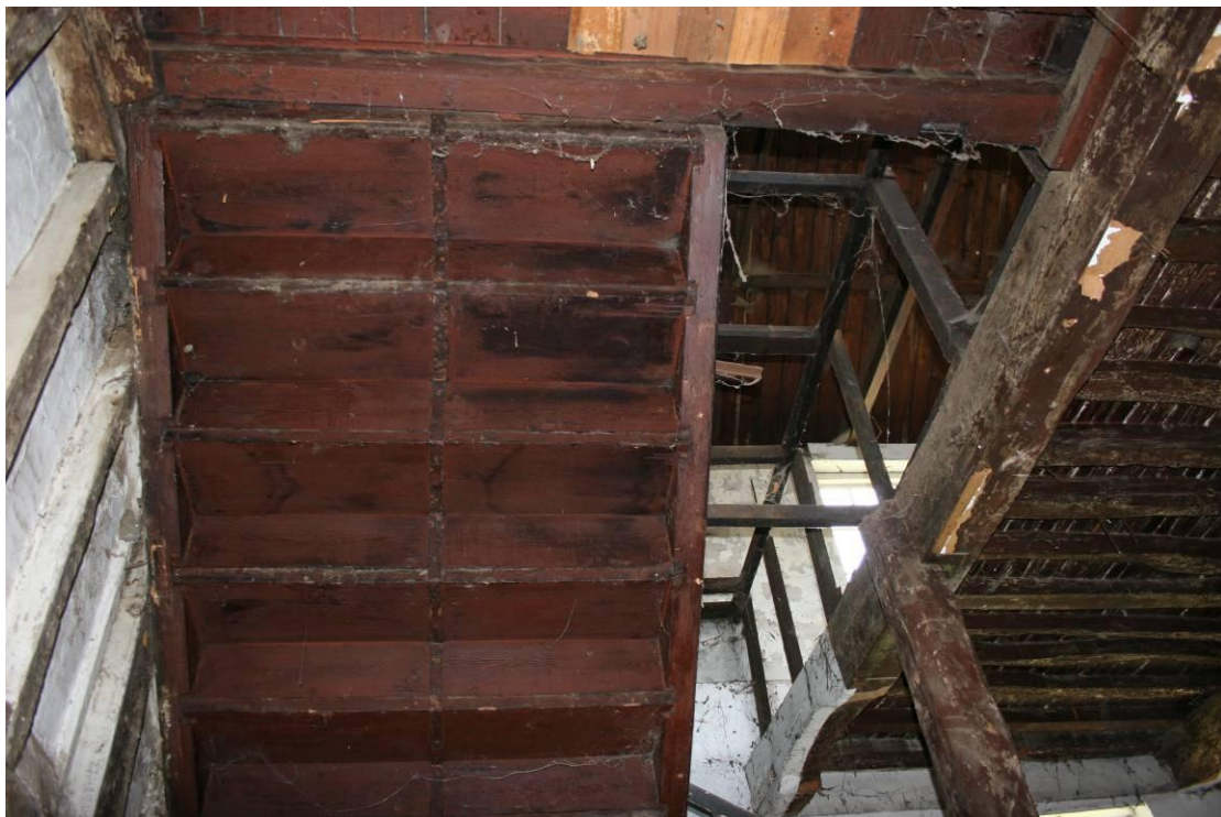
The soffit of the machined treads of the staircase. Looking upwards and E.
