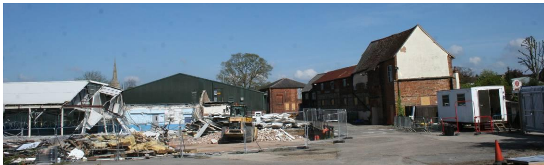
The Listed buildings in context with the factory being demolished. Looking N.
