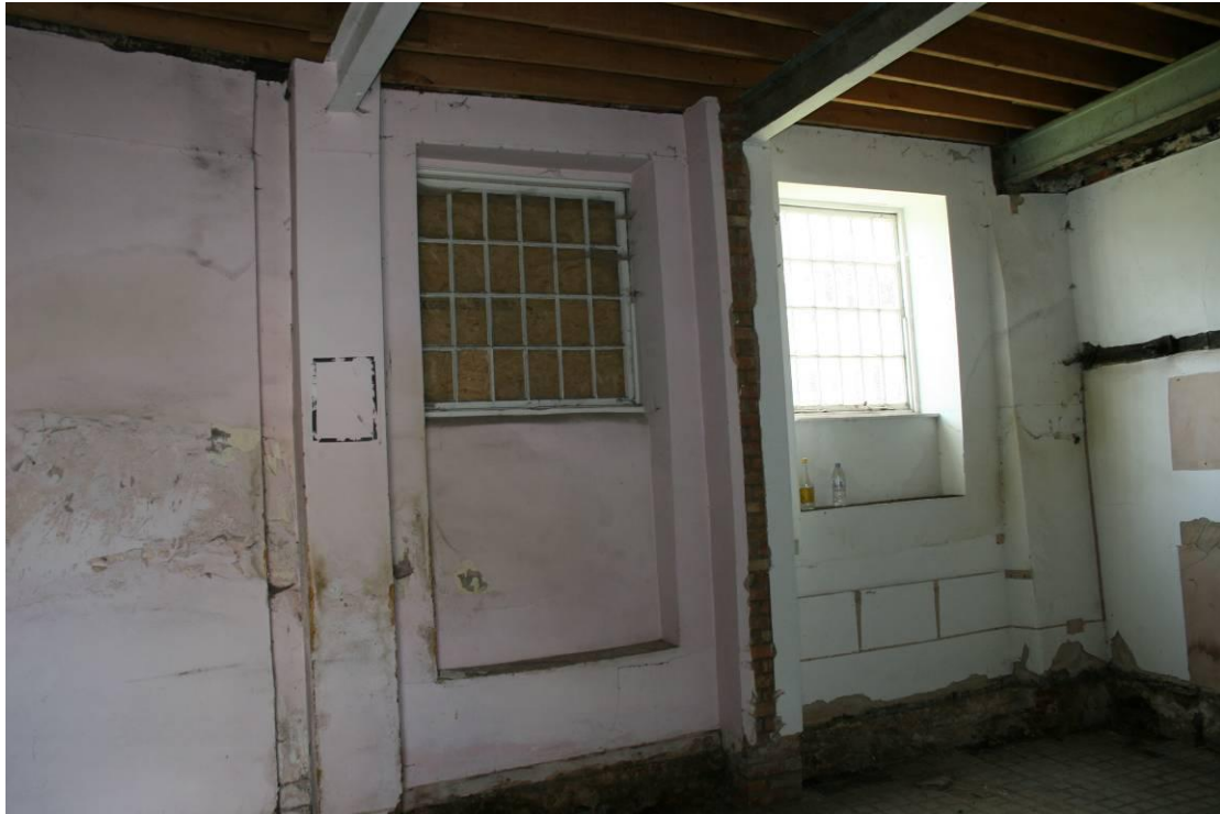
Detail of the blocked doorway and reduced window opening in the eastern wall.
