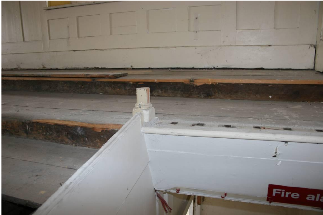
The stump of the newel post and the sockets for the stick balusters.
