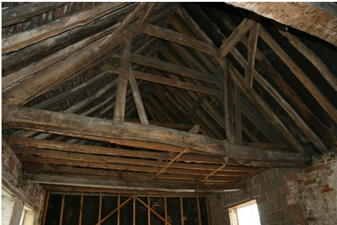
The roof over the southernmost bay beyond the queen post truss. Looking S.
