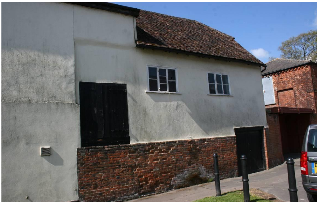
The timber- framed building at the northern end of the range. Eastern elevation.
