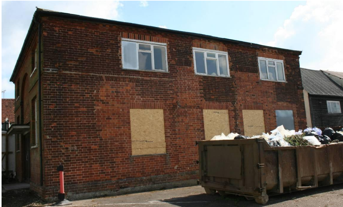
The western elevation. The original brickwork is sooted to a darker red.
