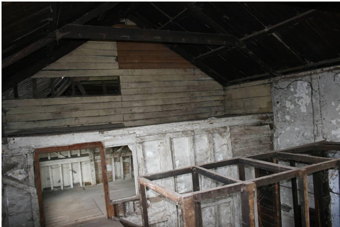
The junction with Building 2 at the northern end of the malting floor.
