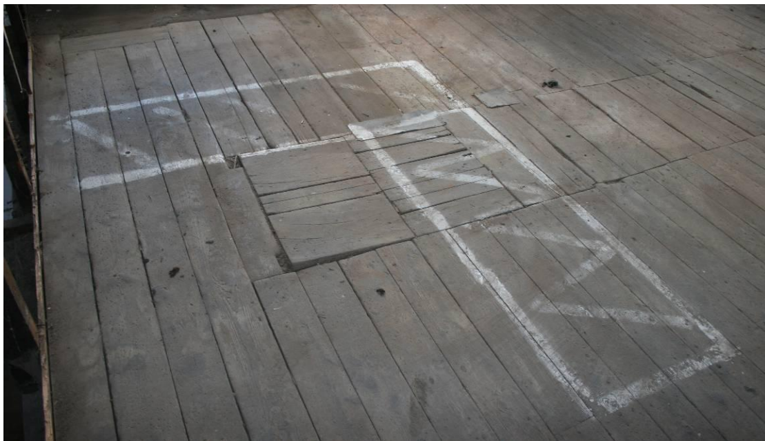
Modern hatch at the northern end of Building 3. The floor was reboarded in the LC19th.
