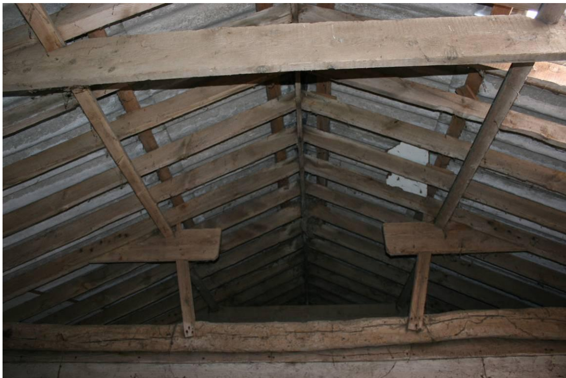
The collar has been cut through and supported on raking struts from the partition wall.
