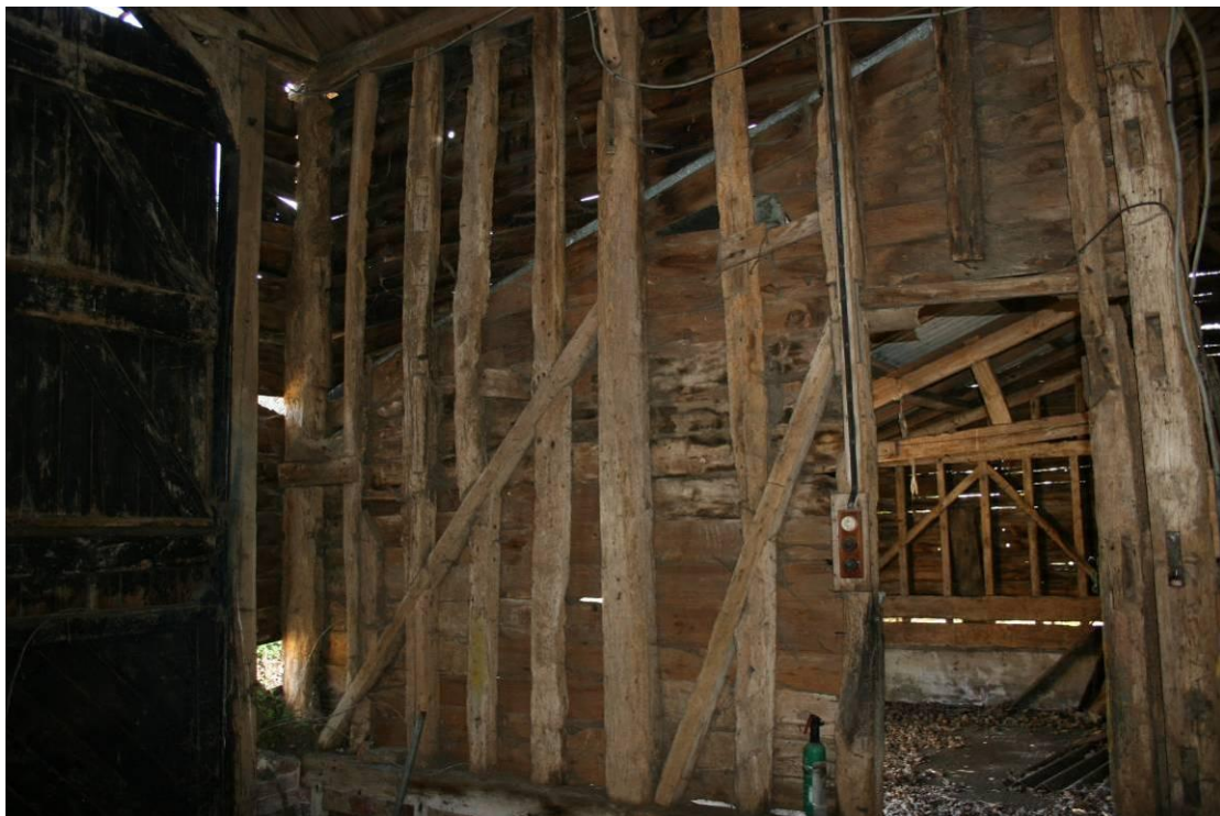
The southern side of the porch. The braces have been designed to accommodate the doorway.
