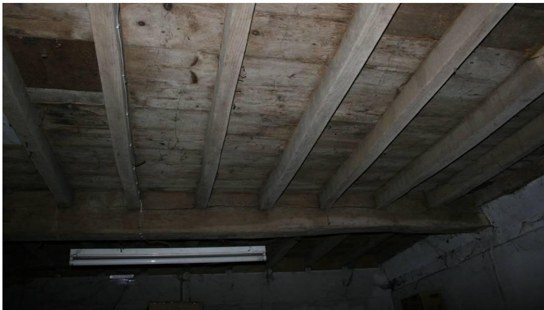
Hatches in the floor allowed the grain to descend into grinding or cleaning machines.
