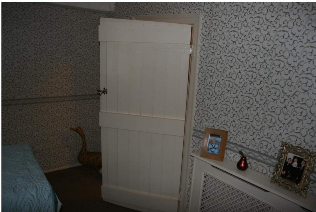
Looking NW in Bedroom 3. An example of a LC20th replica door in an original frame.
