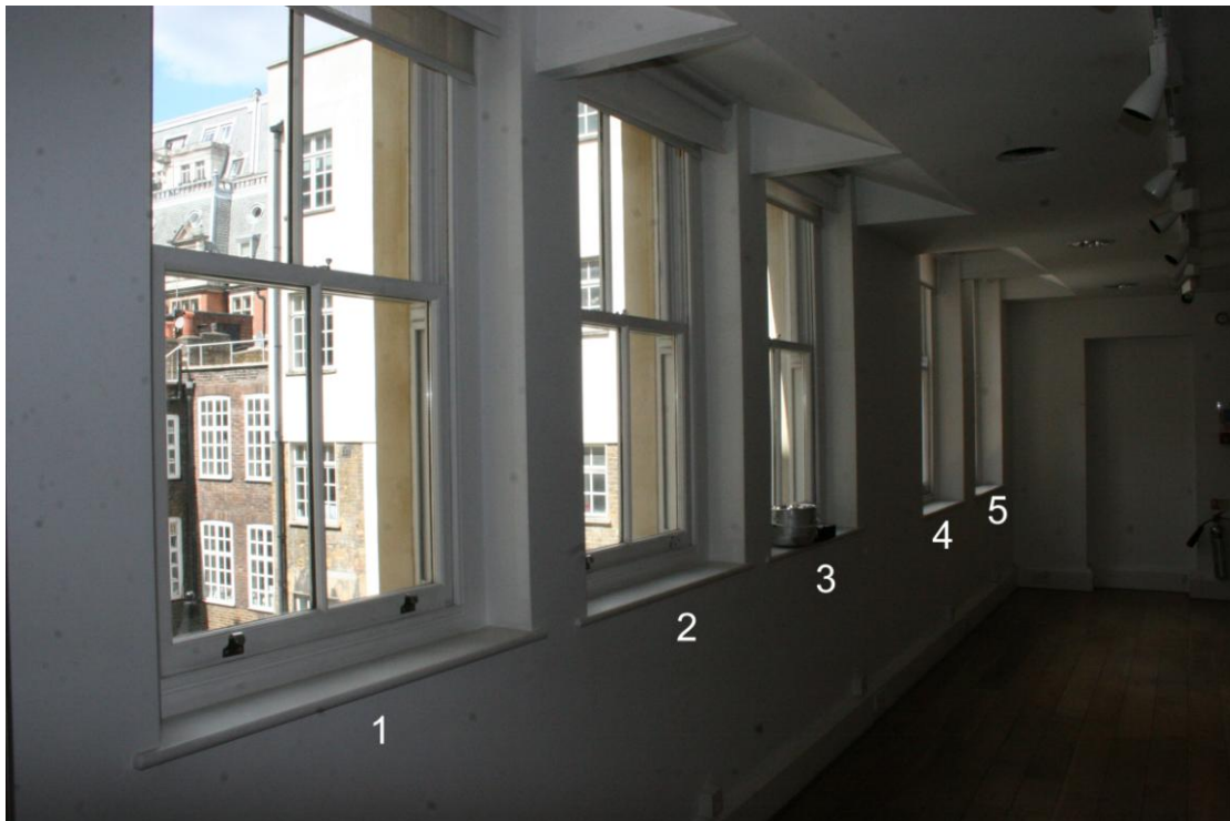
Double glazed sash windows 1-3 have replaced single glazed ones which remain in 4 and 5.
