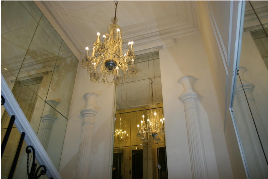
Looking up the staircase from the Ground Floor. The mirror has a door in it.
