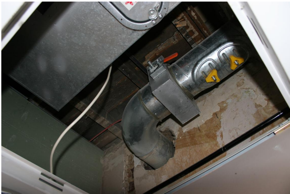
The ceiling and brickwork above the fire hatch
